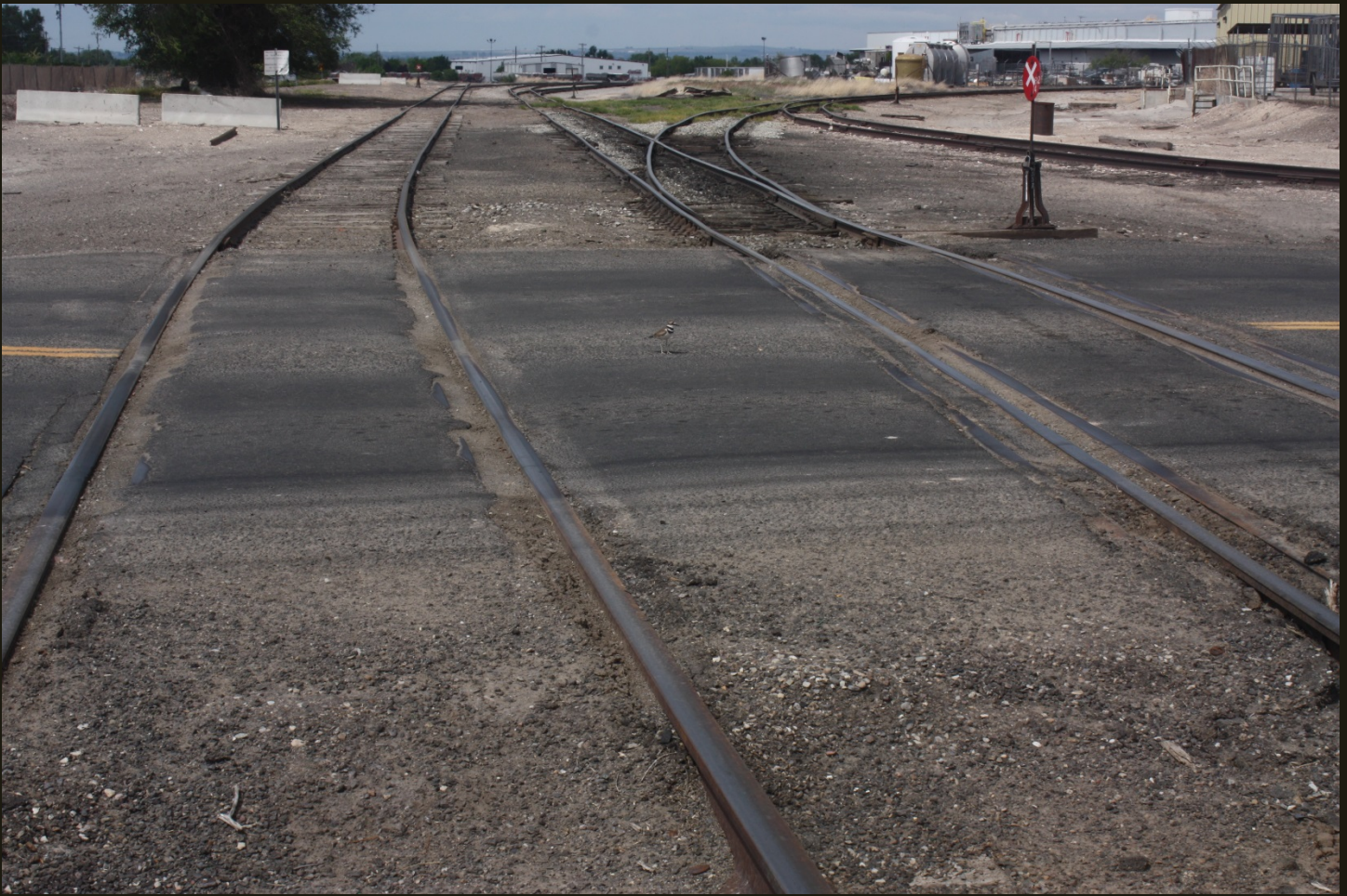
Northward view of the tip of IC Rogerson Branch (1910) wye, 1,400 feet south of previous location. The two branches of the wye converge in the distance then run parallel southward to this location, where they both cross the road in the foreground. The tracks to the right (east) of these two tracks and that connect to the east branch track are short industrial spurs.
