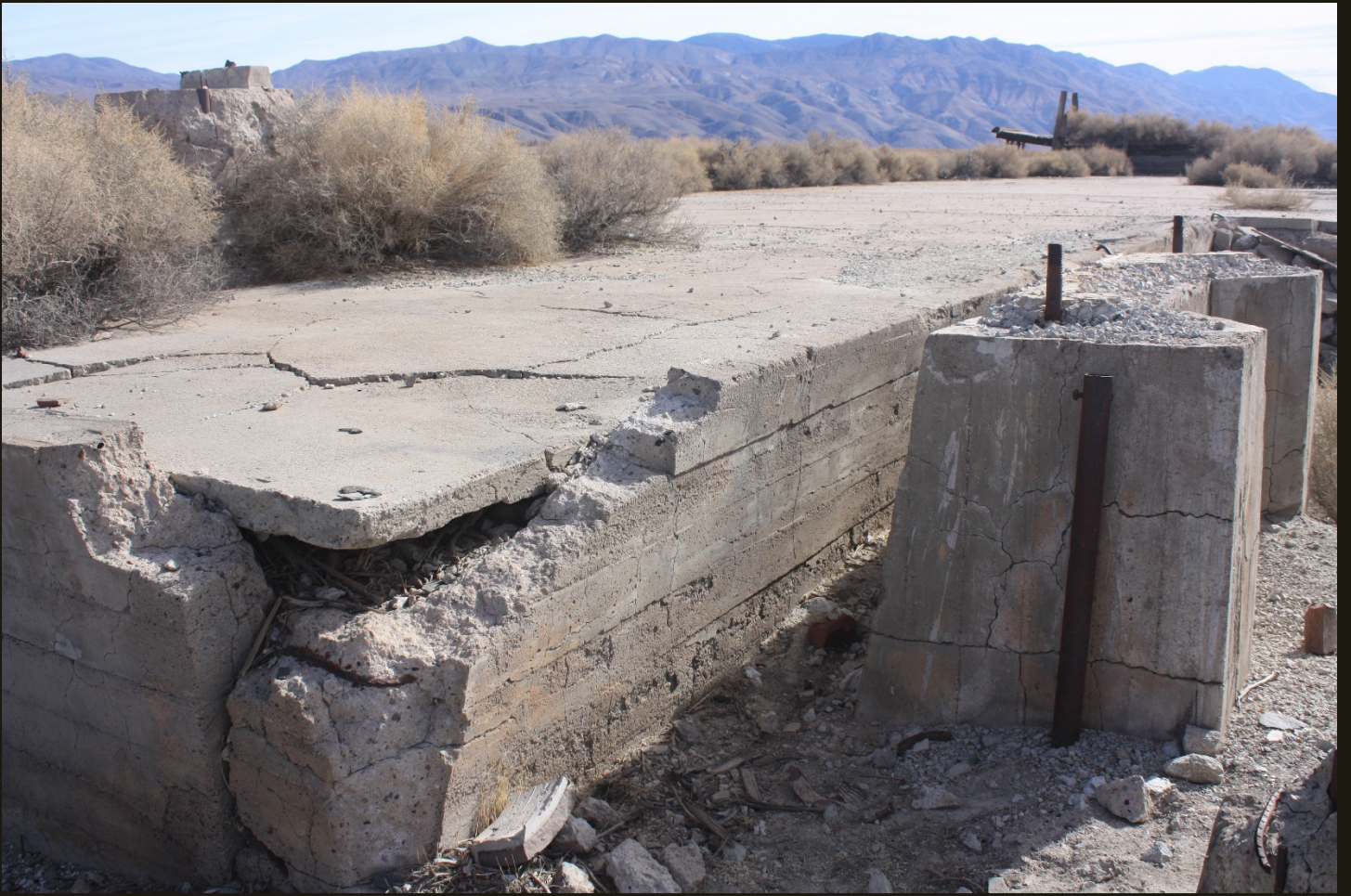
Southeastward view of the foundation of the depot building at Zurich, California. The same post-1960 loading ramp is visible right of center.
