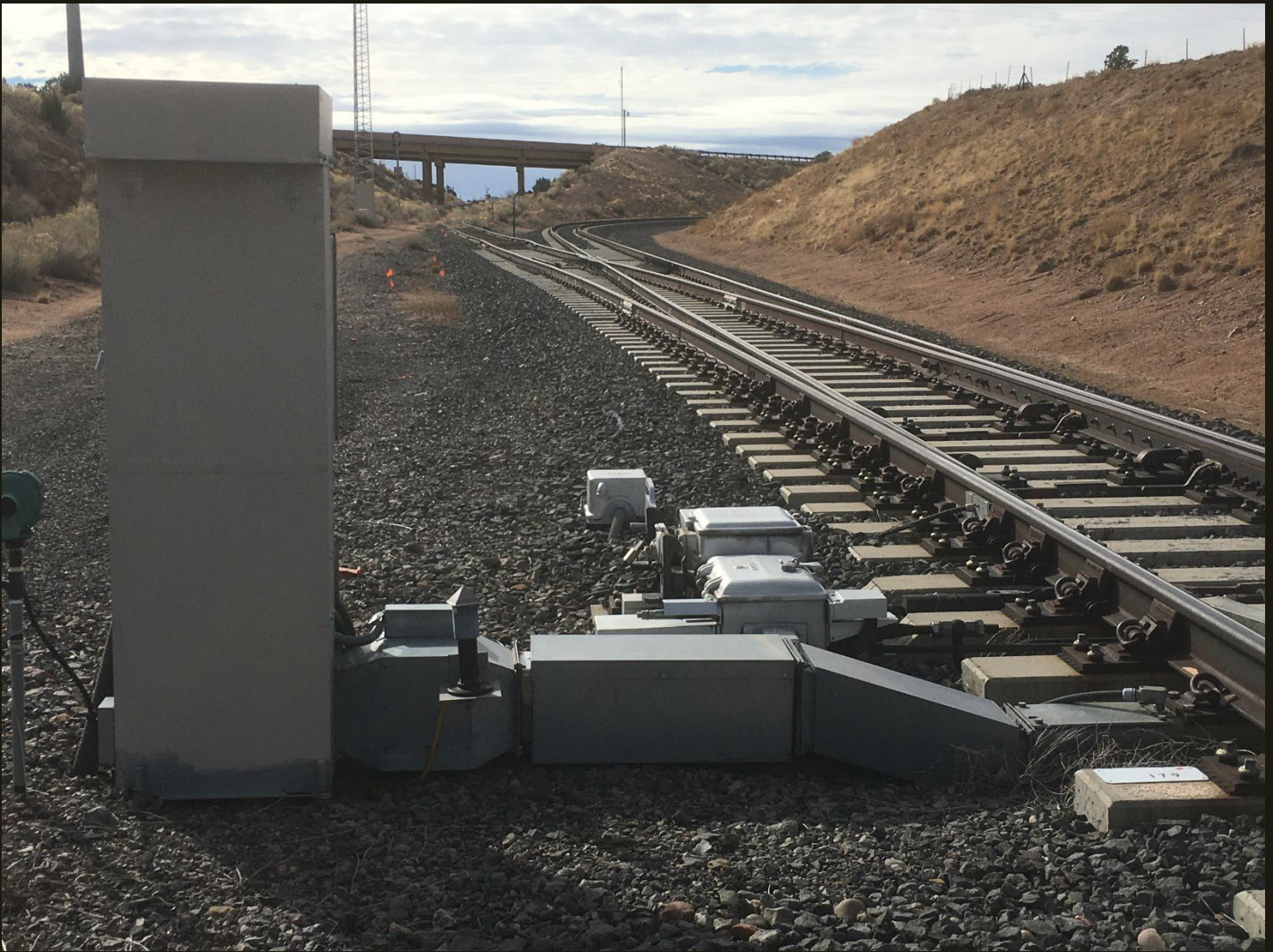
Southward view at the same location as previous. The single track in the right foreground is same track as in the previous photo: the NM&SP Santa Fe Branch (1880) upgraded to concrete ties and welded track for the New Mexico Rail Runner Express. Beyond the switch, the left branch is the non-upgraded NM&SP Santa Fe Branch (1880) to Lamy (on the NM&SP (1881) mainline) and the right branch is a new 2008 alignment for the New Mexico Rail Runner Express.
