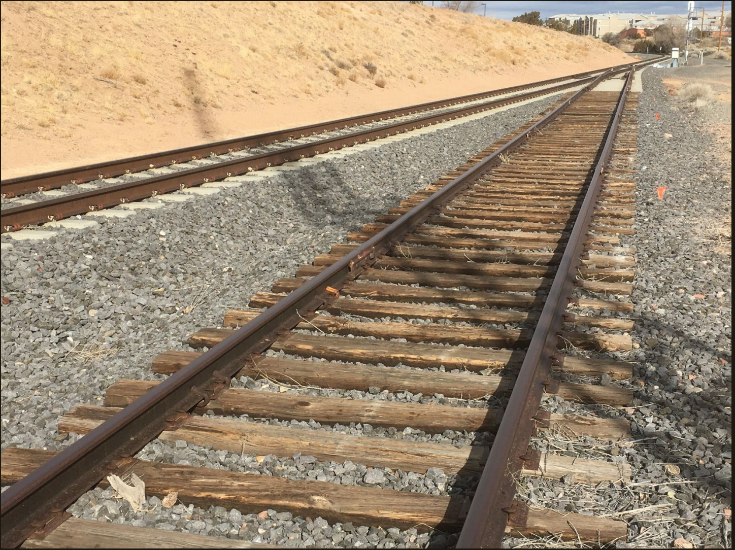
Northward view 300 feet south of the previous location. The non-upgraded NM&SP Santa Fe Branch (1880) is in the foreground with wooden ties and bolted rails and the New Mexico Rail Runner Express (2008) is to its left with concrete ties and welded rail on a new (2008) grade.
