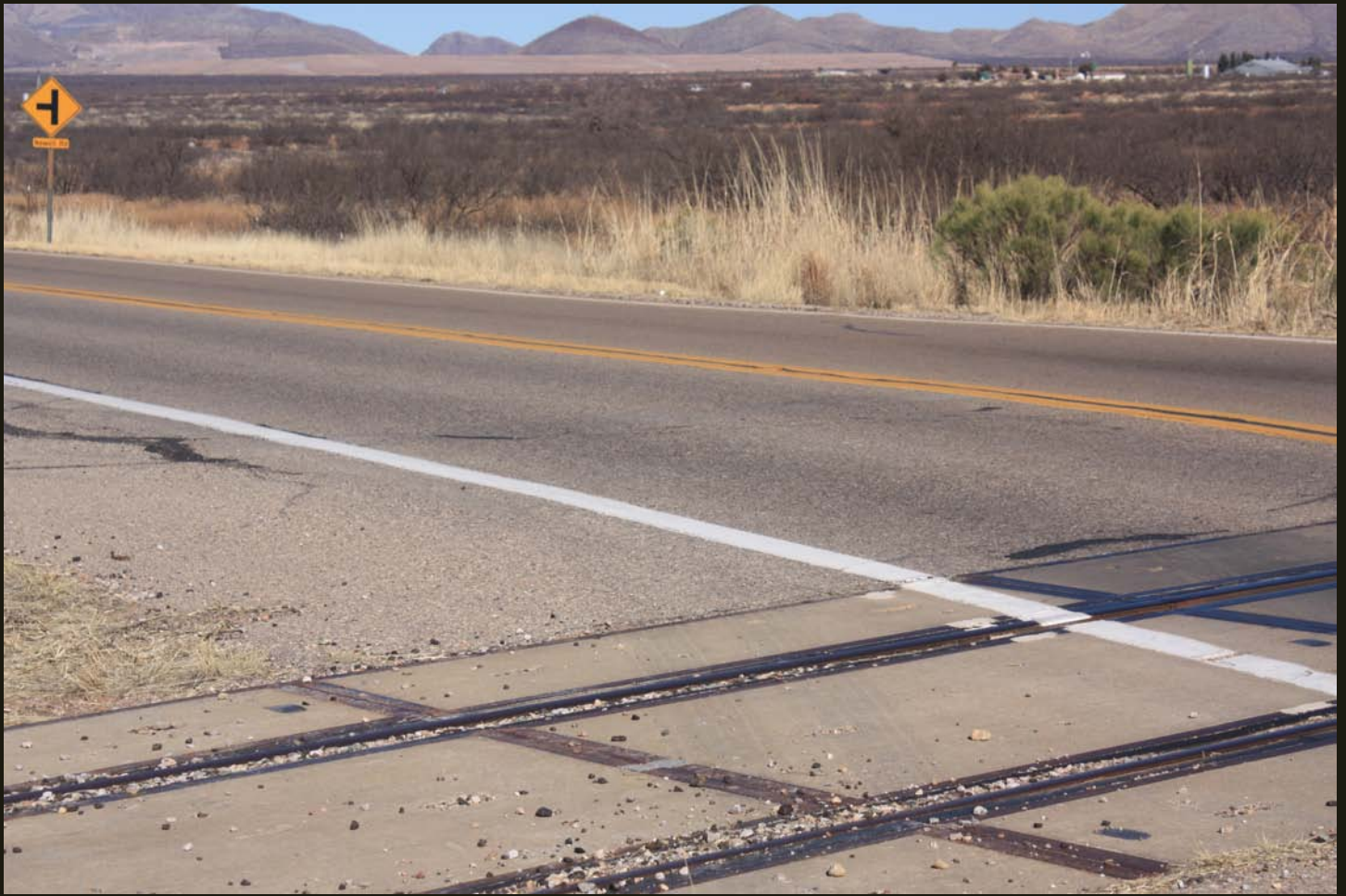
Northeastward view of the EP&SW (1904) where the grade crosses Naco Highway. The tailings pile in the distance is one of several around Bisbee in the Mule Mountains.
