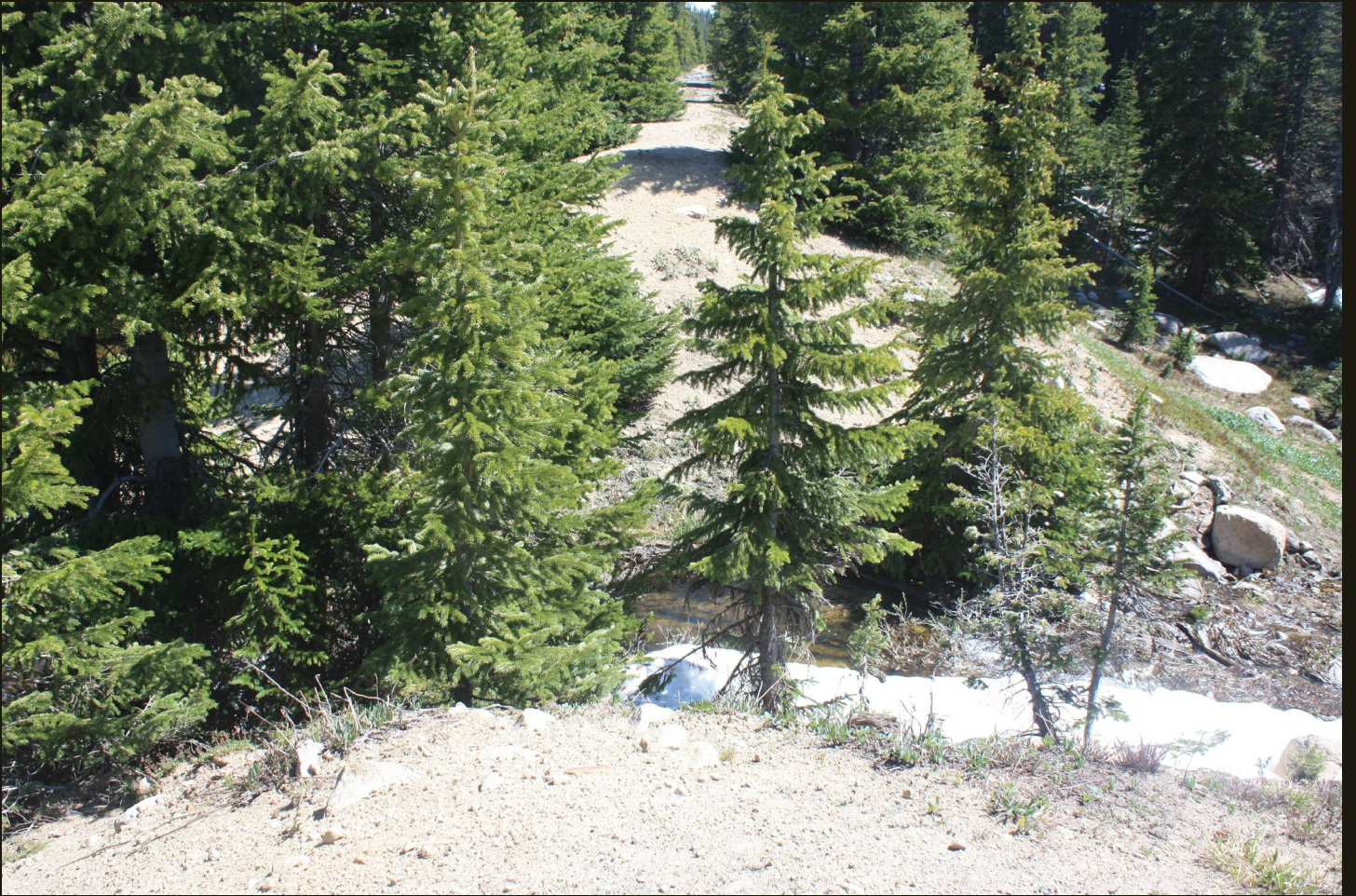
Eroded fill grade on the CM.
