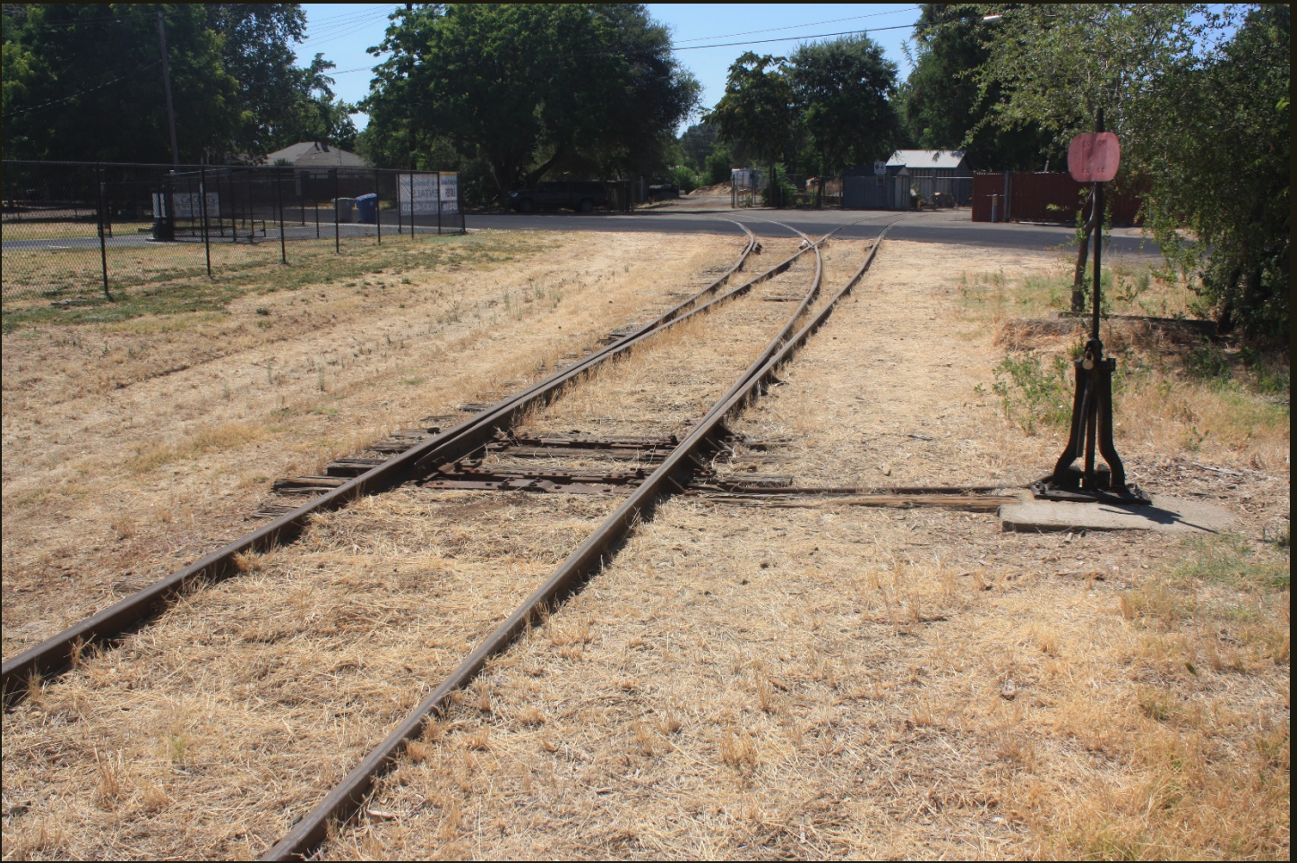
Westward view of the tip of the wye for the S&P (1888), 200 feet east of the previous location.
