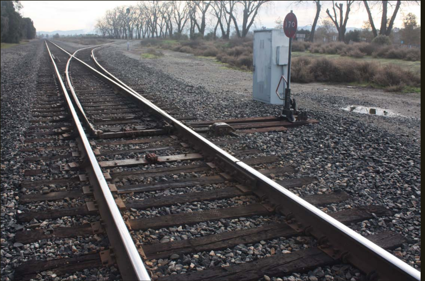
Eastward view of the WP (1909) main line and switch for the Radum siding. The WP (1869) track is in the brush to the right.
