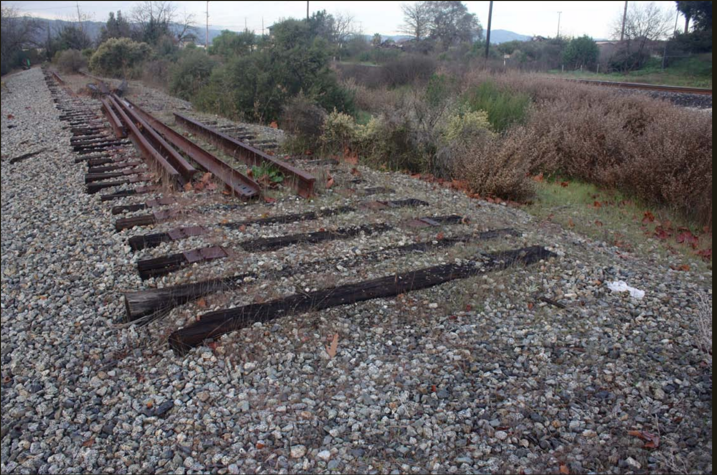
Westward view of partially removed track on the WP (1869) grade. WP (1909) main line in the right distance.
