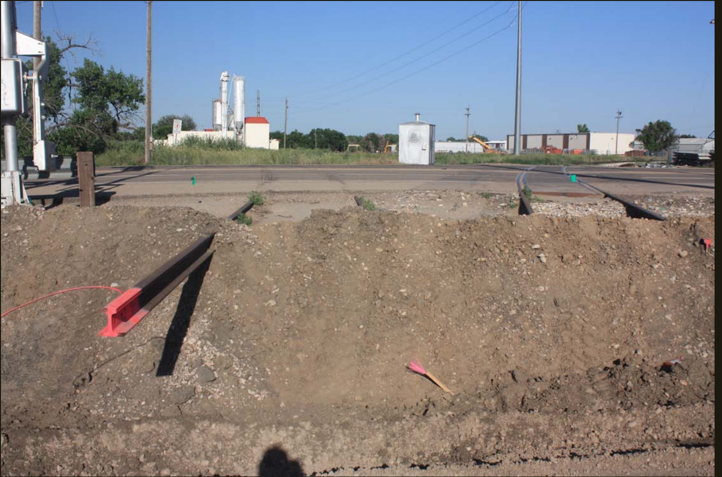
In 2015, tracks were being removed from the Greeley wye on west side of U.S. Highway 85 in this eastward view.
