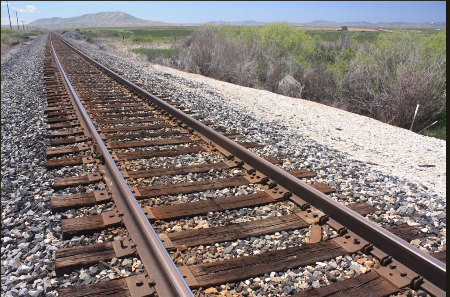
Westward view of the WP (1909), same location as previous, within the Humboldt River marsh. Note the significant fill grade to carry the tracks over the marsh. The curve is the beginning of a broad curve to follow the south bank of the Humboldt River after crossing it and parallel the CP (1869) east to Wells.
