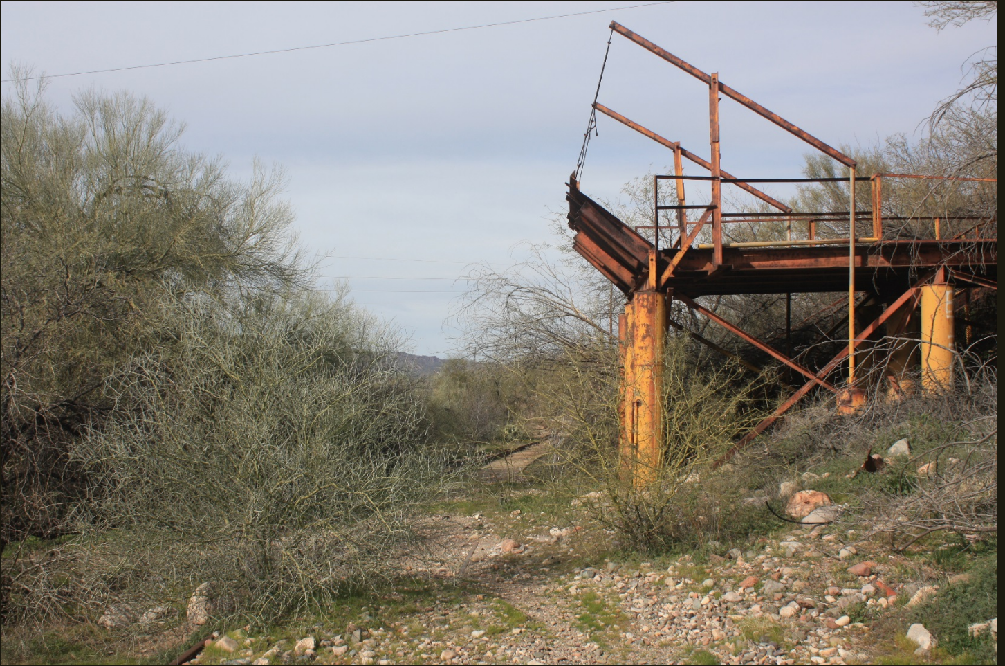
Westward view a few steps east of the previous location, showing details of the loading ramp at Winkelman.
