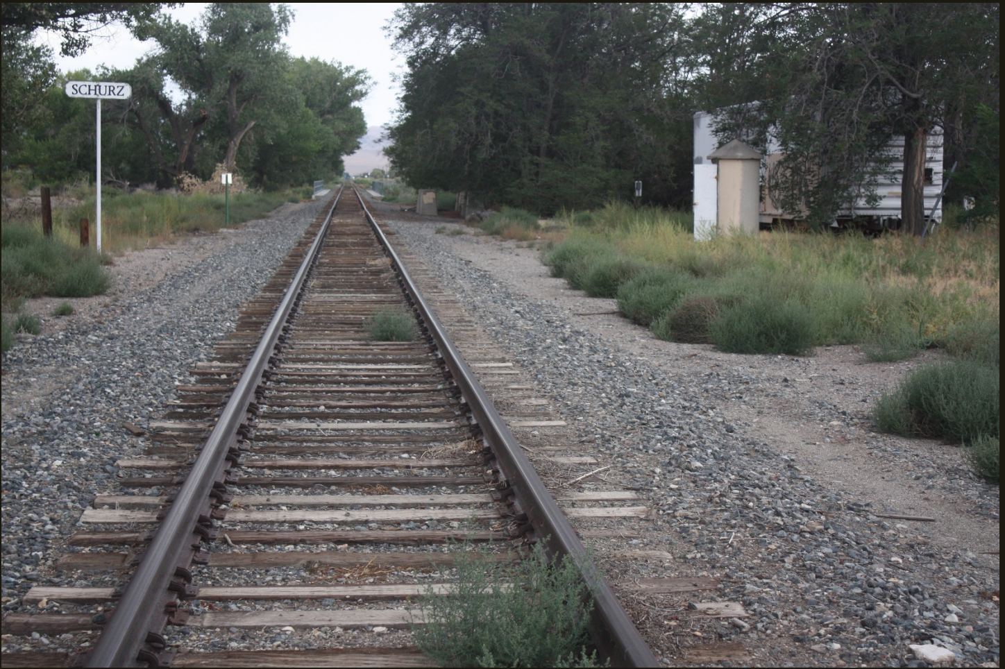
Southeastward view of the C&C (1883n) at the same location as previous.
