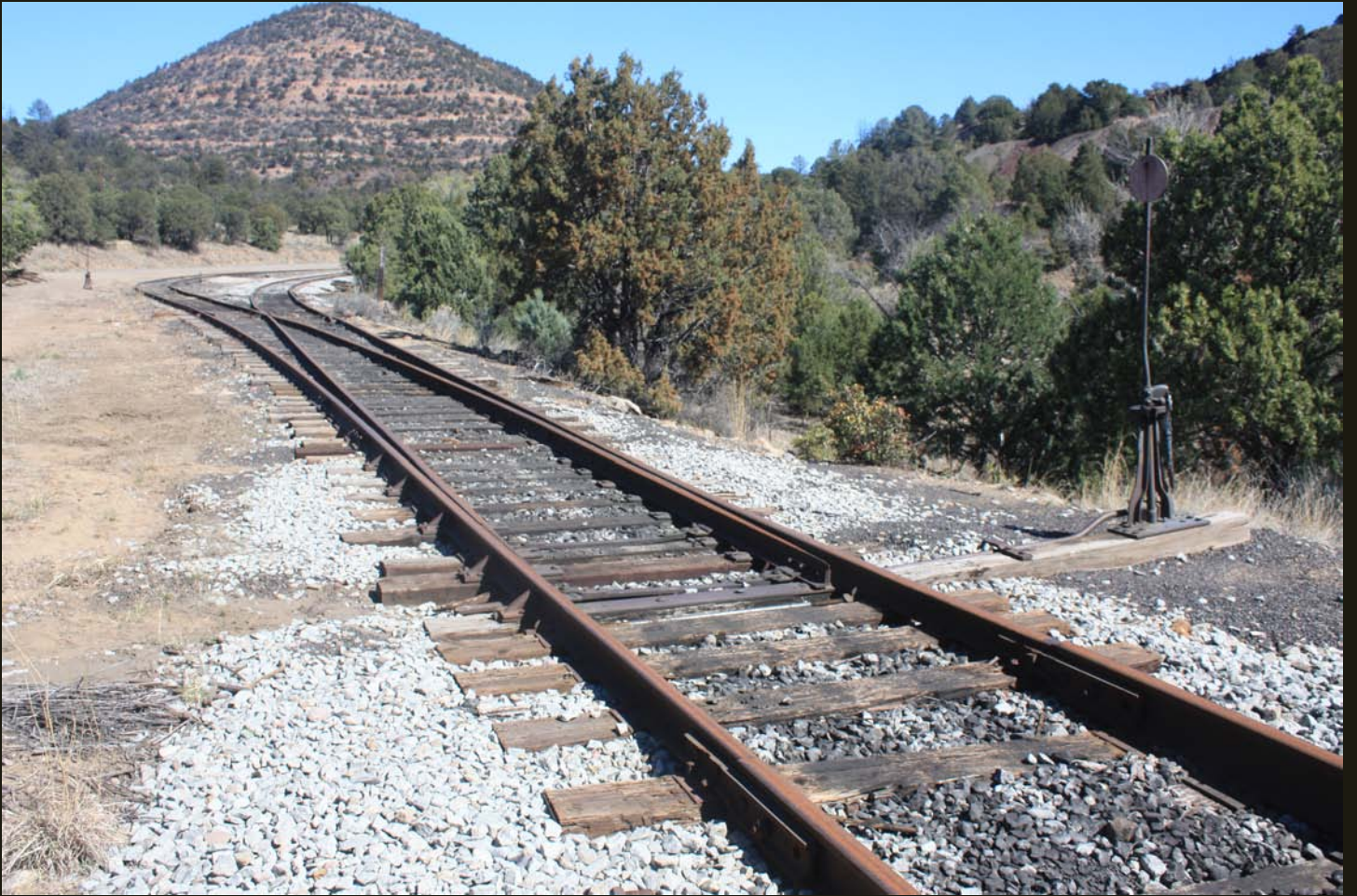
Northward view of the SC&N Fierro siding. Heavier rails in the foreground change to lighter rails at the switch (see next photo).
