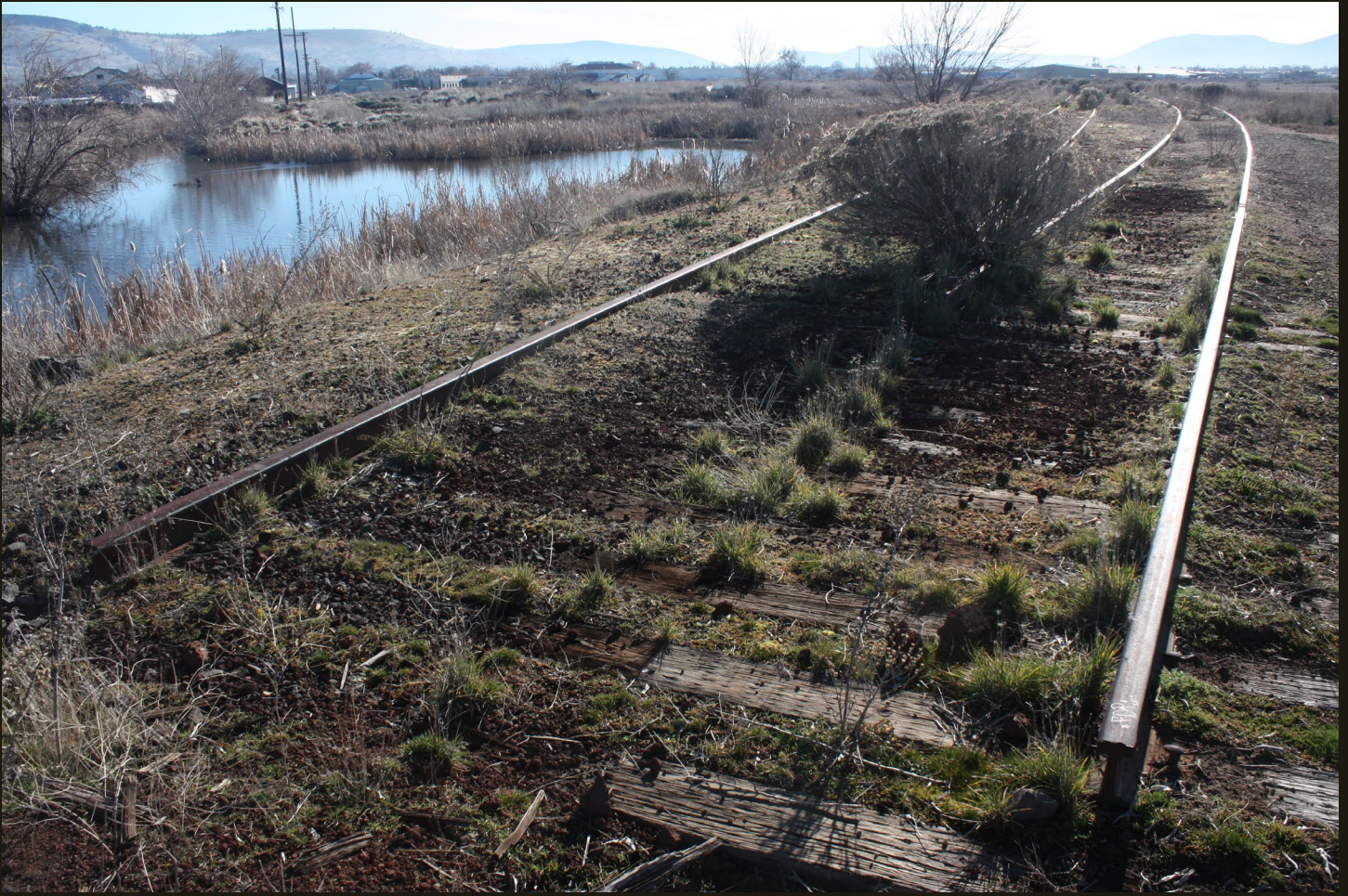
The current (2015) end of track on the OC&E (1923) grade, just a few feet from the active C&NE/UP mainline. There was a switch for a siding here, and double tracks extend about a half mile to the east, where the tracks end and the grade east is now the OC&E Woods State Trail.
