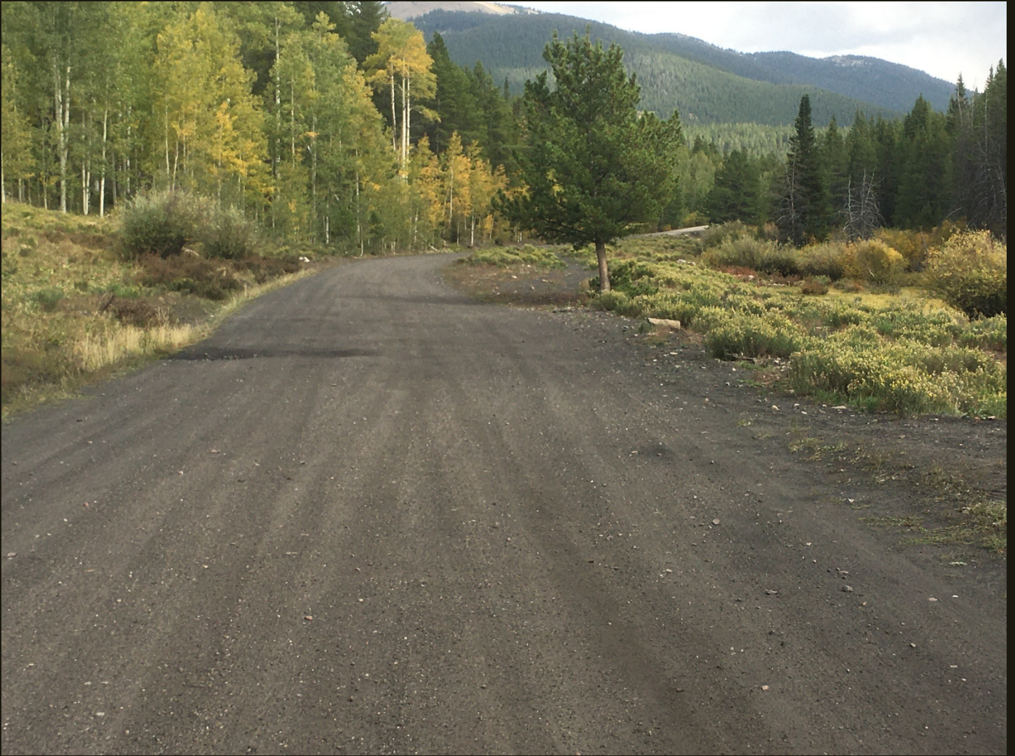
Northwestward view of the CM (1888) 2.75 rail miles upgrade from the previous location. The lower part of the CM (1888) is only 0.4 miles to the left (southwest).
