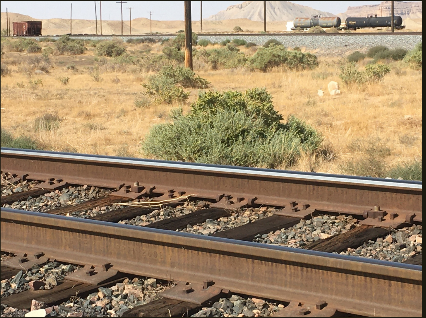
Northwestward view of the Cane Creek Branch (1963) at the same location as previous, showing the same stored cars as before.
