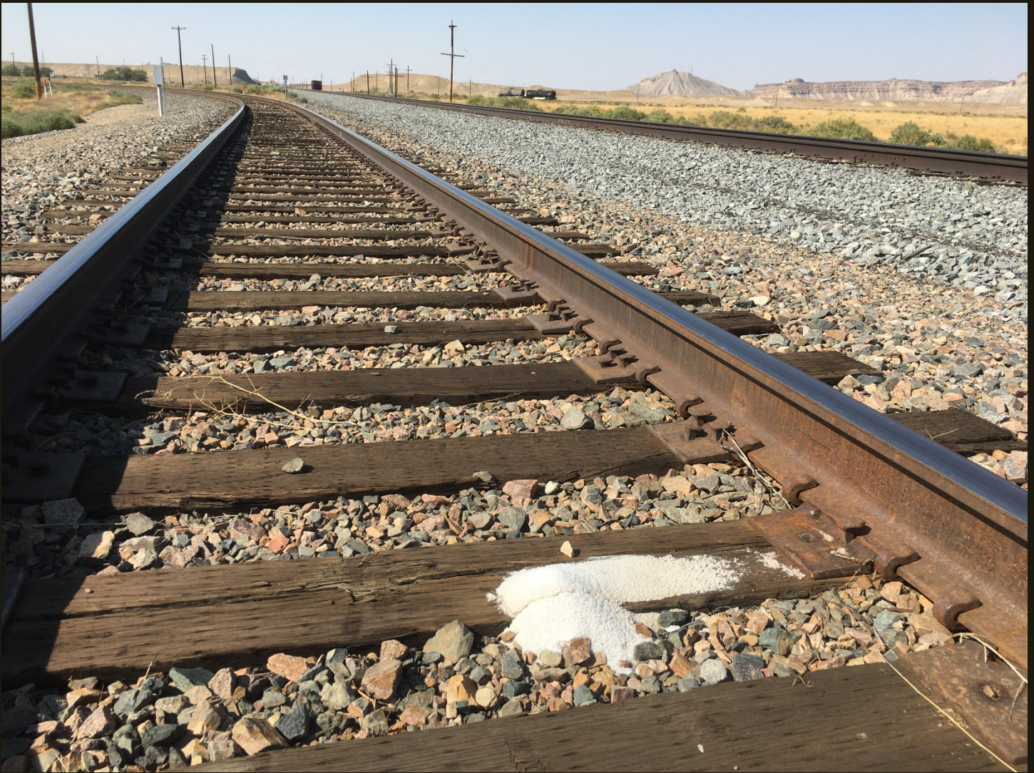
Westward view 1,000 feet west of the previous location. The welded-track Cane Creek Branch (1963) is in the foreground, with some spilled potash on the track, beyond which the alignment begins its left turn to the south. In the distance, note the stored car on the siding next to the mainline and the two stored tank cars that seemed to be out in the desert.
