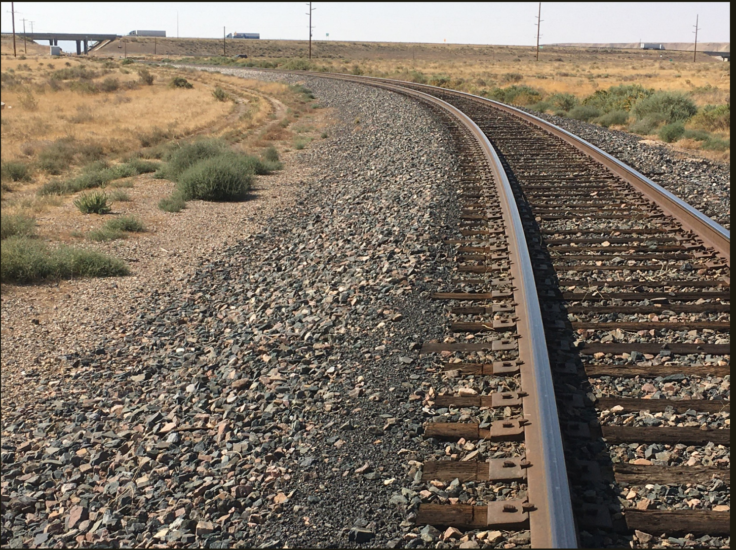
Southwestward view at the same location as previous, as the Cane Creek Branch (1963) continues its curve to the south. Note the overpass for I-70.
