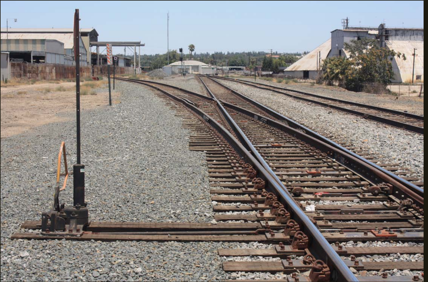
Northward view of the MS line and sidings; the wye with the SP (now UP) is in the distance.
