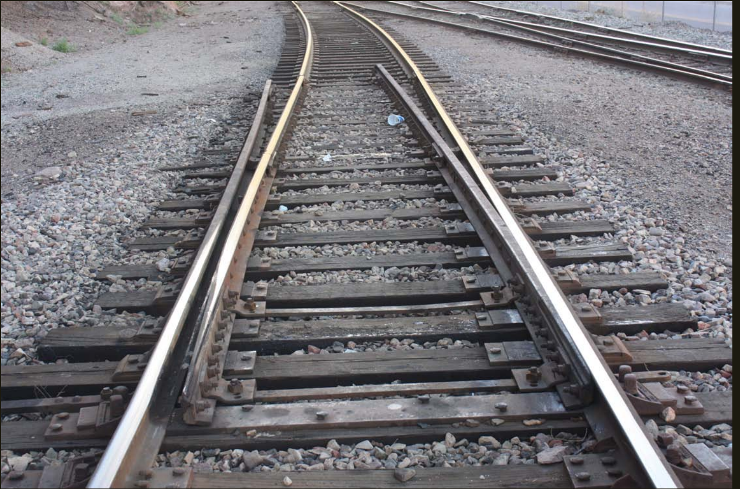
Closer view of the open switch at the base of the MS grade.
