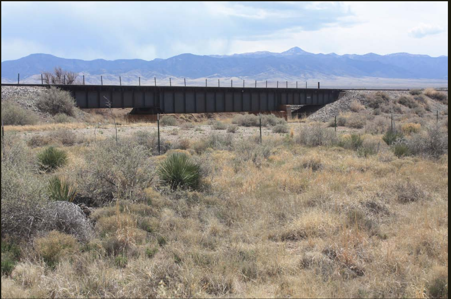
A small bridge carries the EP&RI grade over a wash 5 miles north of Carrizozo. This bridge may be original 1901 EP&RI construction, but more likely was an upgrade by a successor, either the EP&SW, Southern Pacific, or Union Pacific. The Sacramento Mountains are in the distance.
