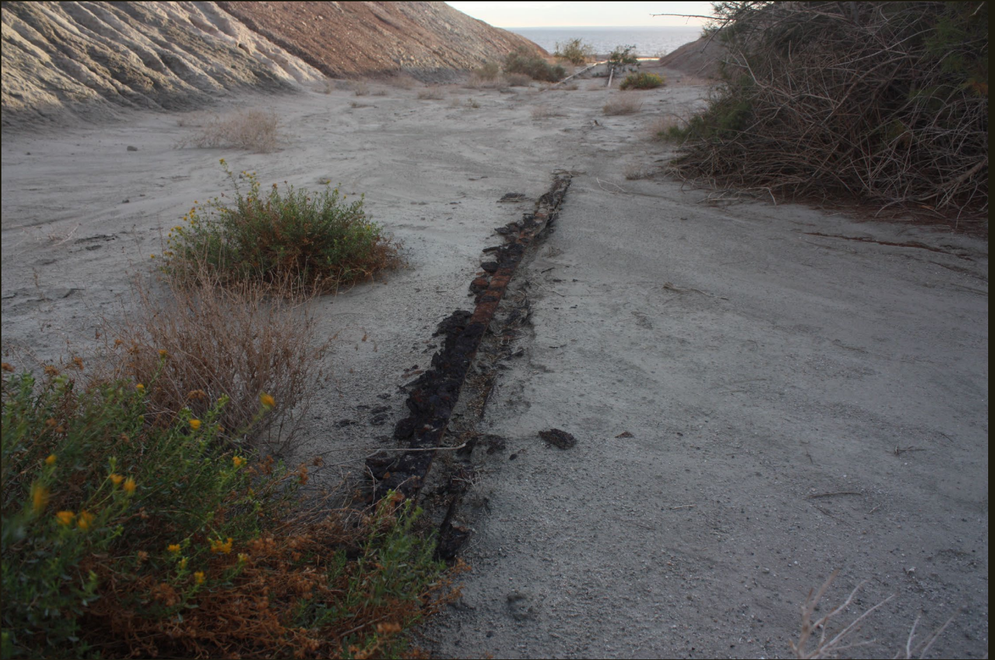
Westward view of the Ferrum turning wye. Track is partly buried by erosion of the cut grade; heavy rusting in the foreground.
