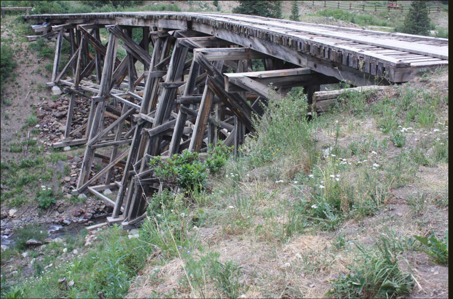
This trestle negotiates the Lake Fork of the San Miguel River, the last stream crossing south of Lizard Head Pass.
