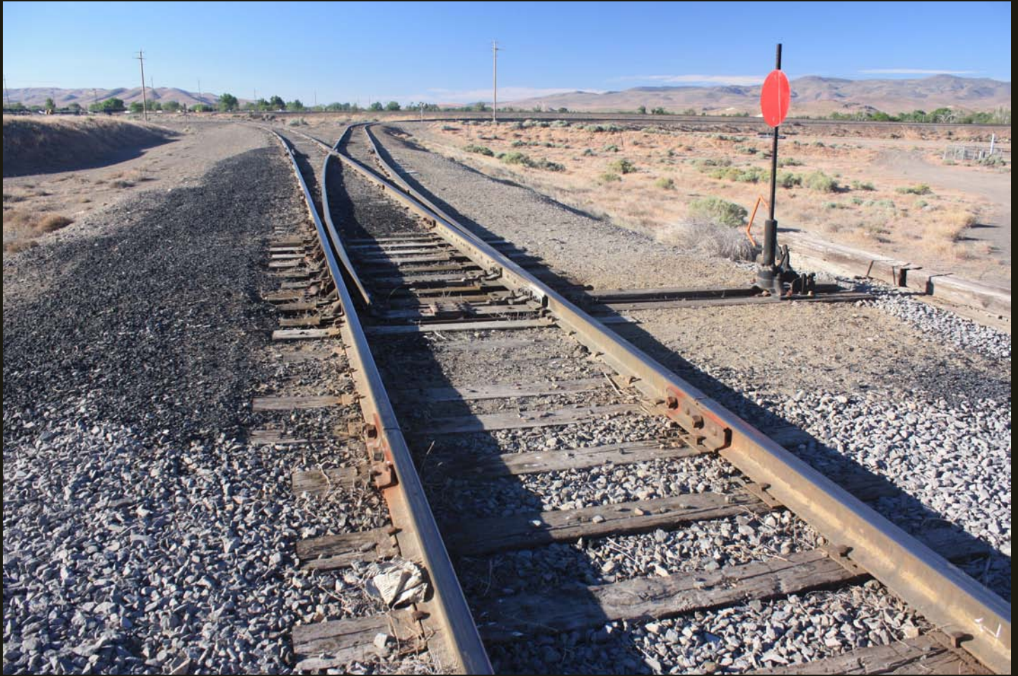
Southward view of the F&L (1914), same location as previous at the north tip of the wye for its connection to the SP (1902) re-alignment at Fernley. The SP (1902) re-alignment is barely visible in the distance between the two branches of the wye.
