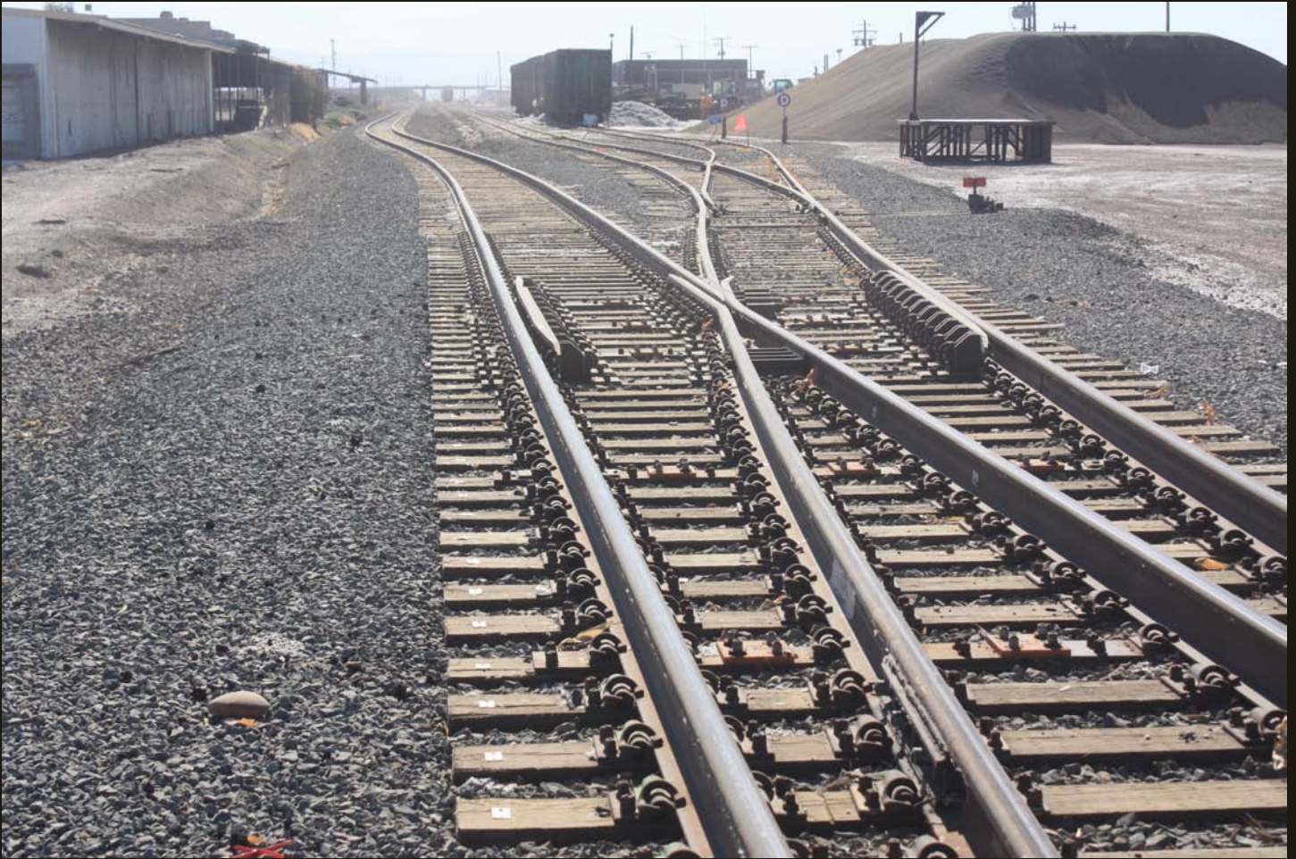
Another westward view of sidings and loading facilities on the SW just west of the Connor 90. Note piled cotton, ready for transport over the RailAmerica-owned San Joaquin Valley Railroad, which plies the remaining western half of the SW (1909).
