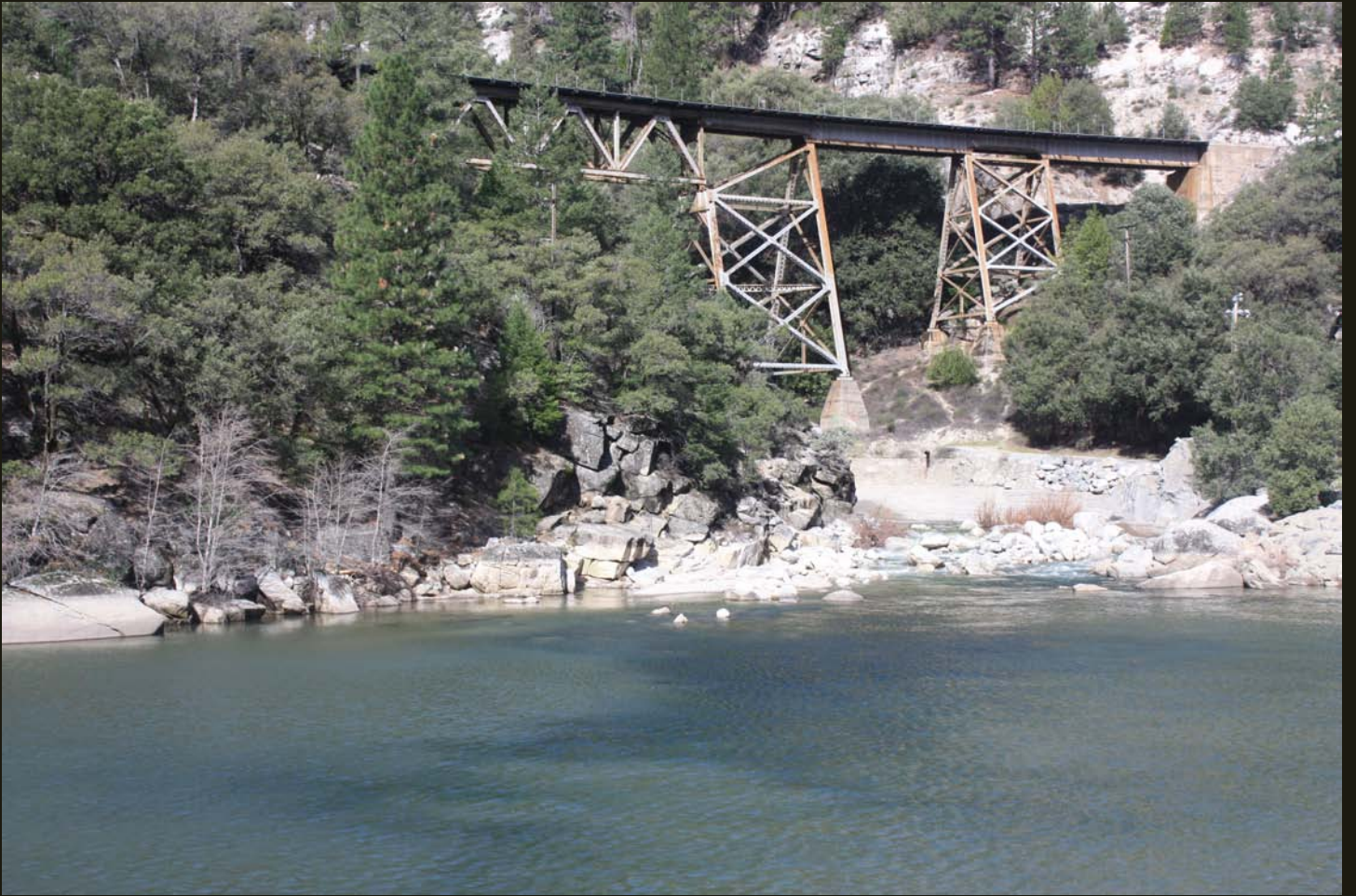
A trestle carries the WP over a tributary of the North Fork Feather River.
