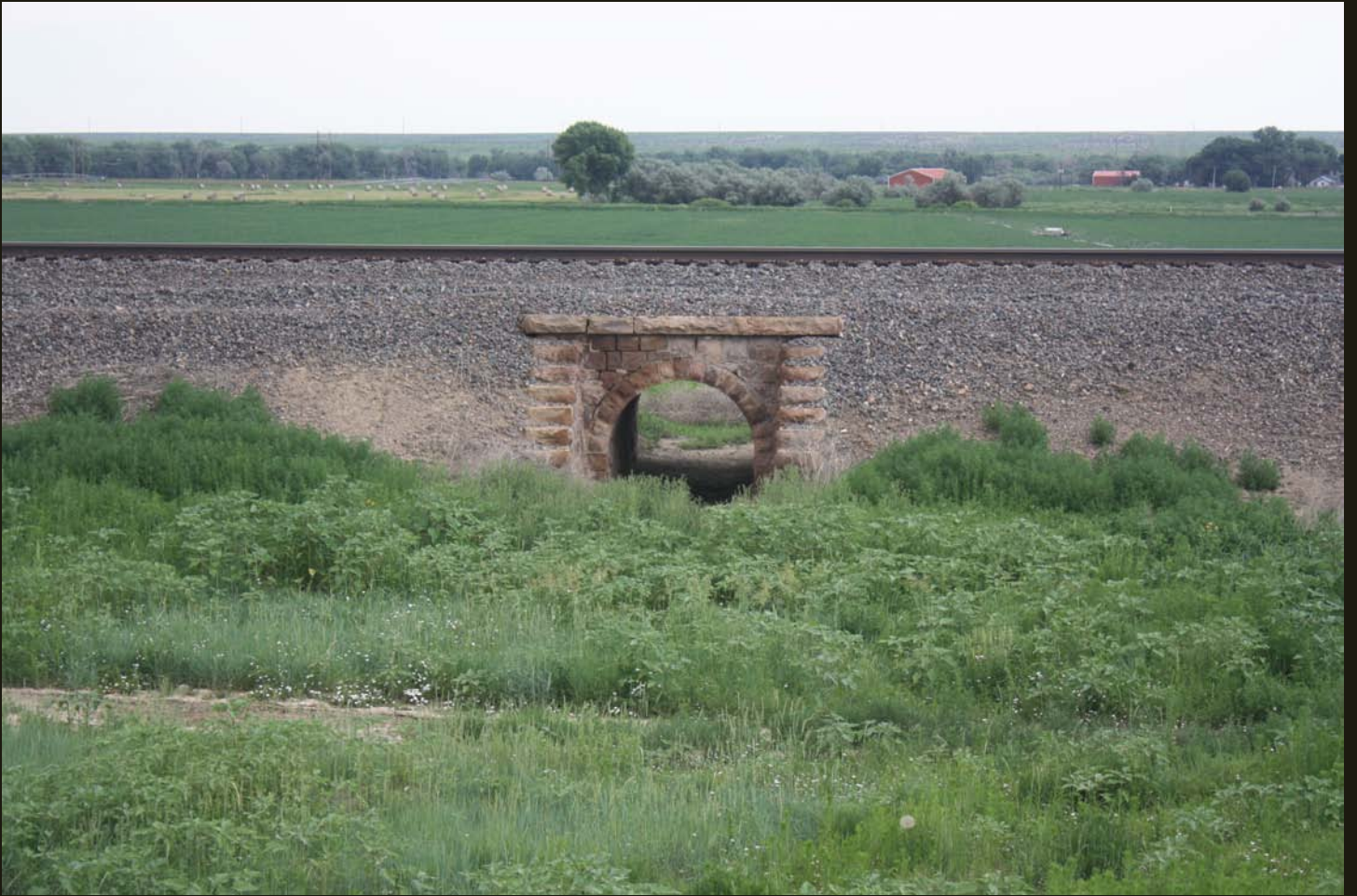
This small culvert on the D&RG is work of art in itself.
