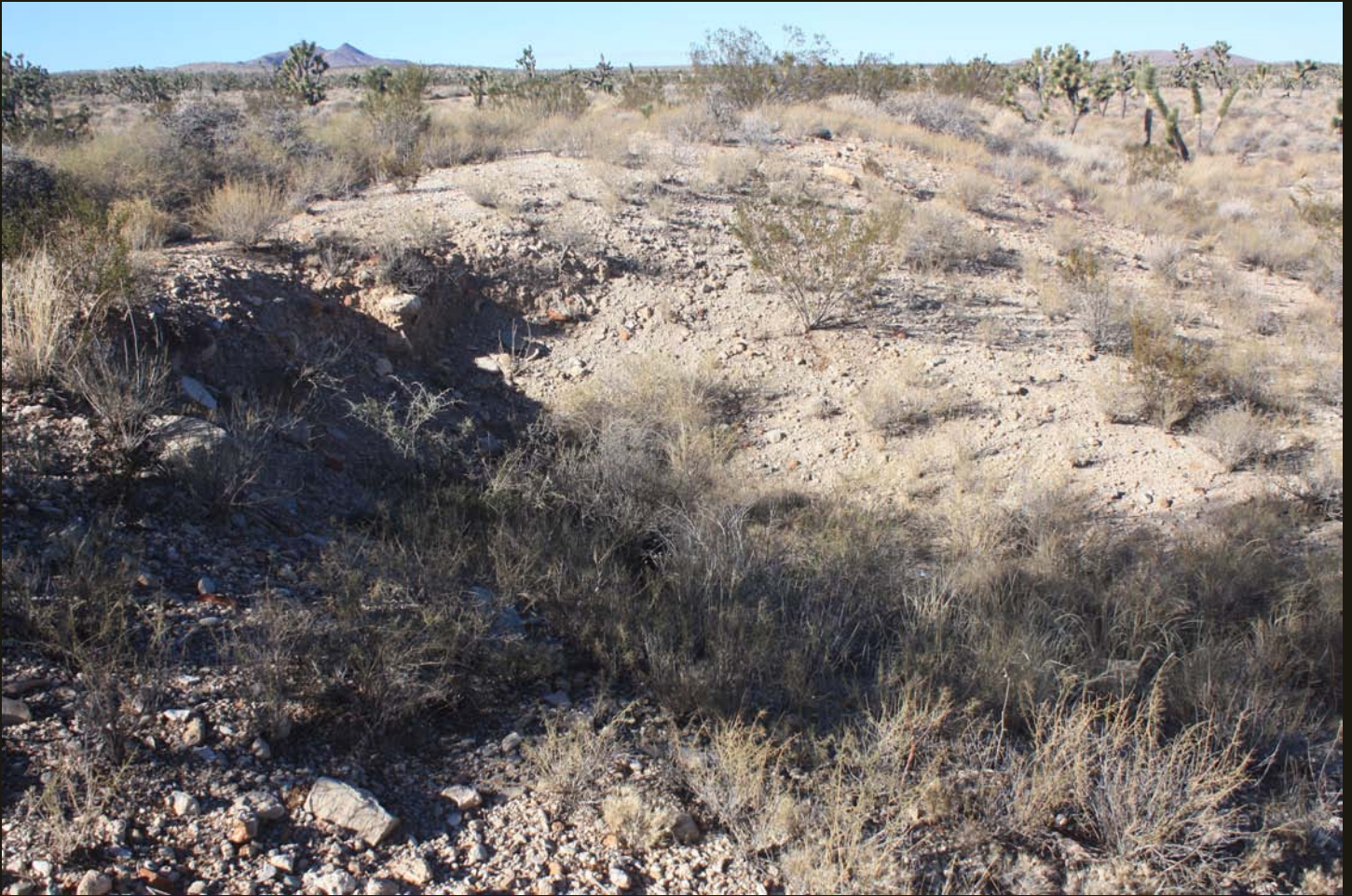
Northward view of the NS grade, 5 miles north of the previous location on the 1893 5-mile extension to Manvel/Barnwell. Note the washout of the fill grade in the foreground, one of many.
