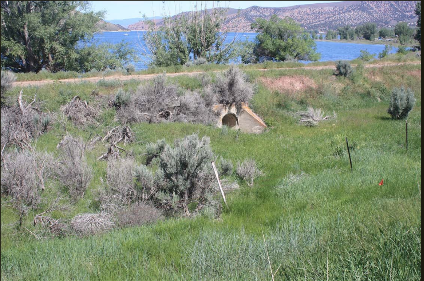
The E-PC grade 4 miles south of the UP mainline at Echo. Note the culvert to allow runoff to flow under the grade. Echo Reservoir, an impoundment of the Weber River, is in the background.
