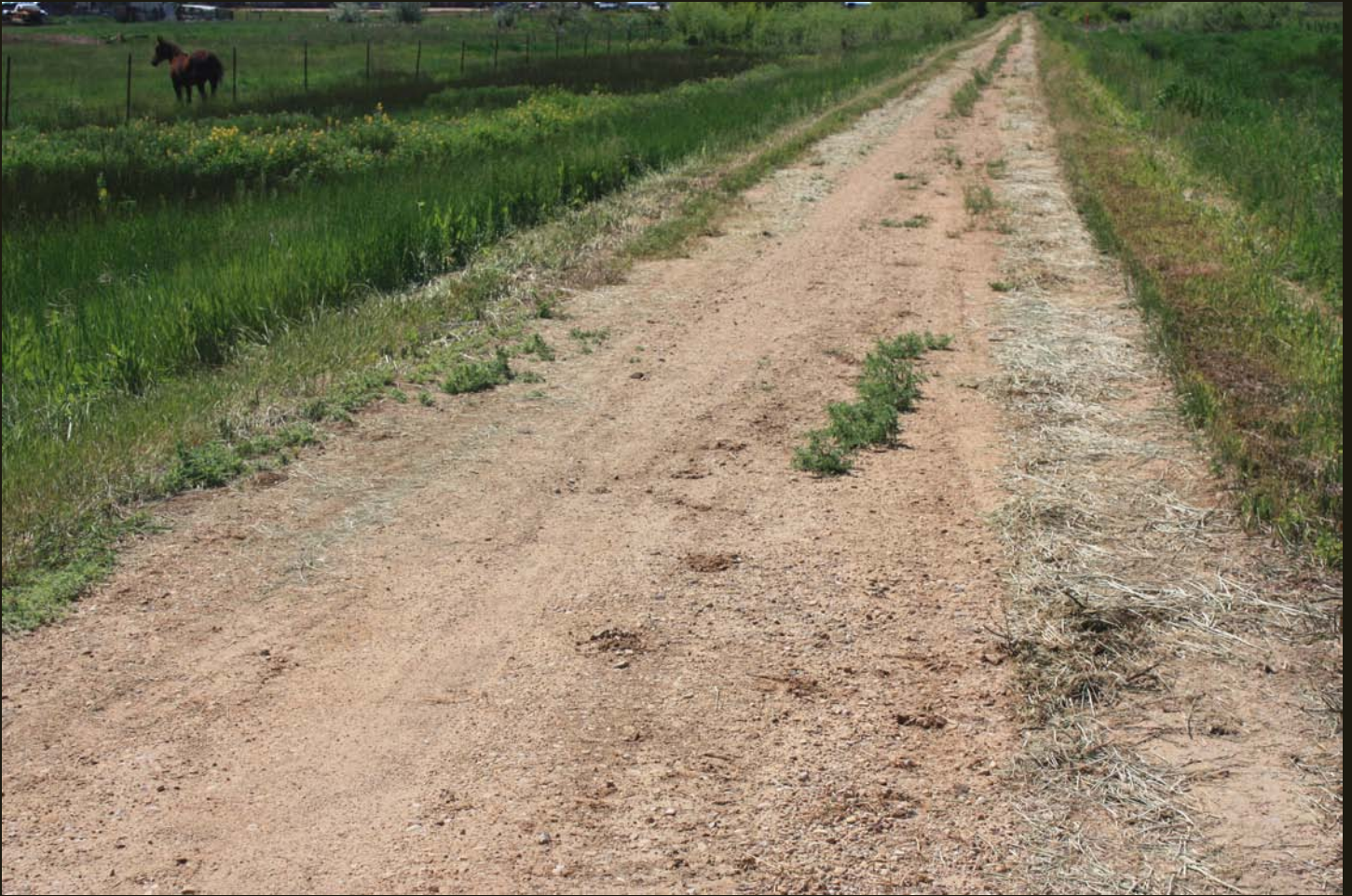
The E-PC grade 5 miles south of the UP mainline at Echo. The grade crosses wetlands along the Weber River just south (upstream) of Echo Reservoir.
