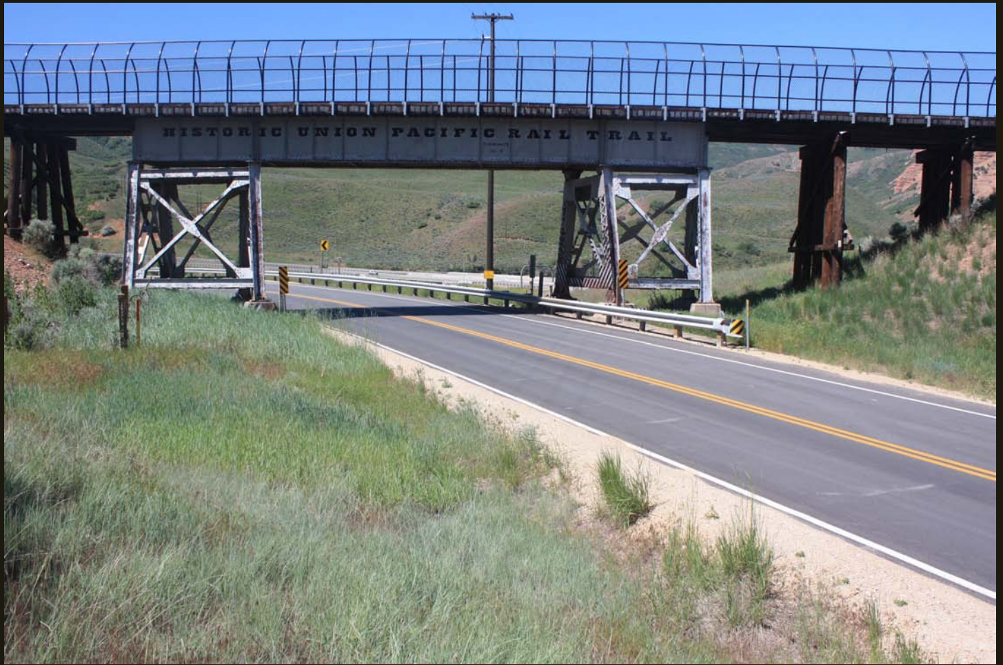
This steel and wood bridge carries the E-PC over a road near Echo, Utah, and is now part of the Historic Union Pacific Rail Trail.
