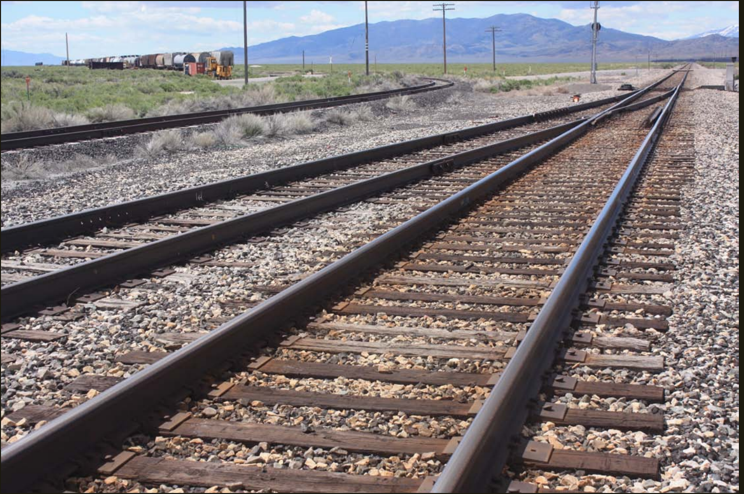
Southwestward view of the WP (1909) and NN (1906) at Shafter. The original grade crossing was just past the WP signal, where the WP goes to one track. The NN is completely gone north of the crossing (to the right of the WP tracks). The curved trackage to the left connects to the NN south of the former crossing and the cars are on the NN (1906) alignment.
