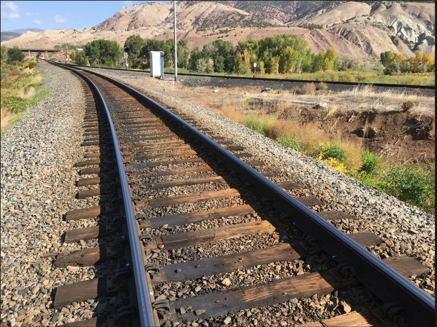
Northward view of the west branch of the wye 300 feet north of the previous location, where it converges with the east branch in the left distance. The I-70 crossing of the D&RGW Dotsero Cutoff (1934) is in the left distance and this completes our clockwise tour of the Dotsero wye.
