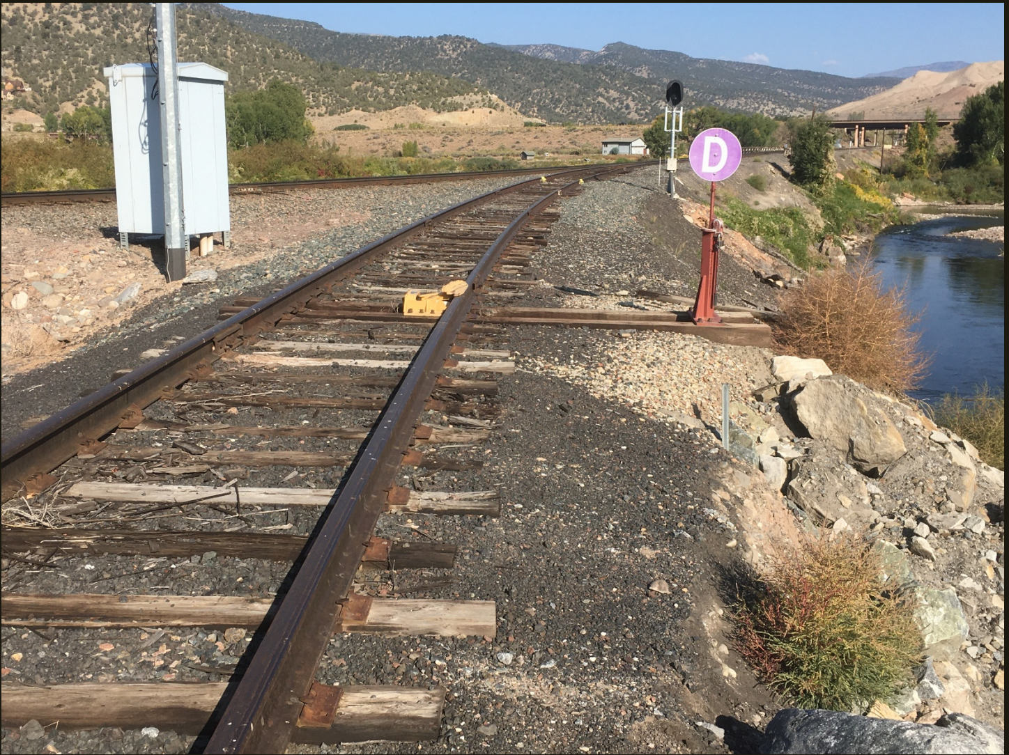
Northwestward view of the east branch of the Dotsero wye. The west branch of the wye is on the left, the Eagle River is on the right, and the same overpass for I-70 is in the distance. The derailing device at the switch may have been there since the 1990's to prevent trains from heading towards Tennessee Pass on unmaintained tracks.
