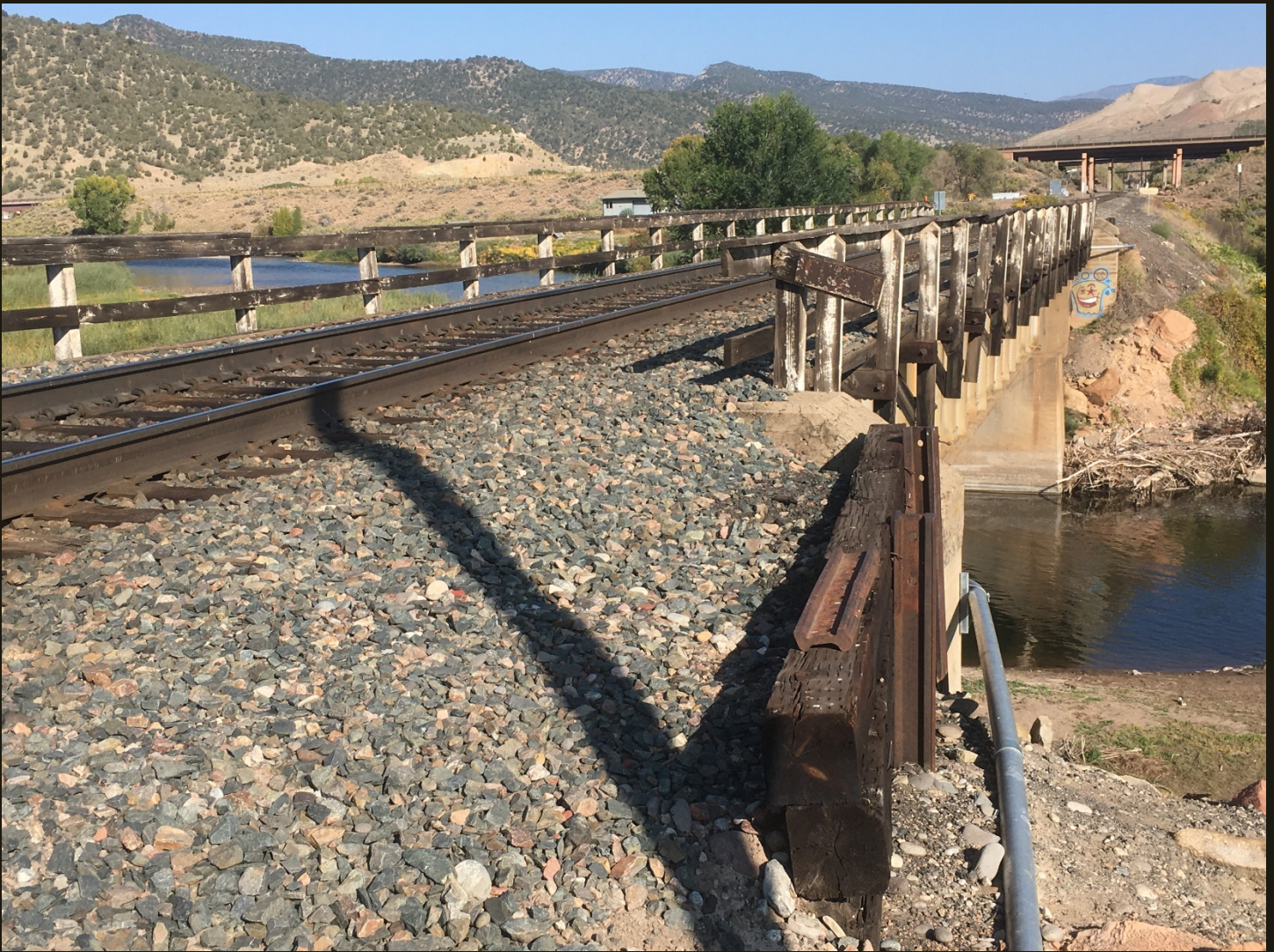
Northward view of the D&RGW Dotsero Cutoff (1934) just north of the north tip of the wye. The bridge crosses the Eagle River, which flows into the Colorado River on the left.
