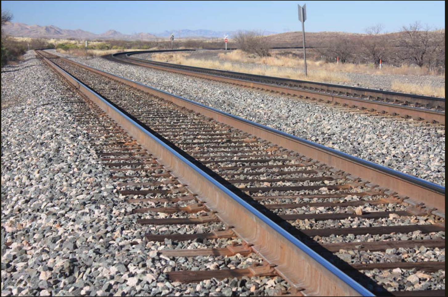
Westward view of the SP/UP double track one mile west of Mescal. The track to the left continues into the distance on the SP (1881) alignment. The track to the right is a 1920's vintage crossover that joins the EP&SW (1912) alignment just out of sight to the right and uses the EP&SW (1912) for 20 miles before the two routes rejoin.
