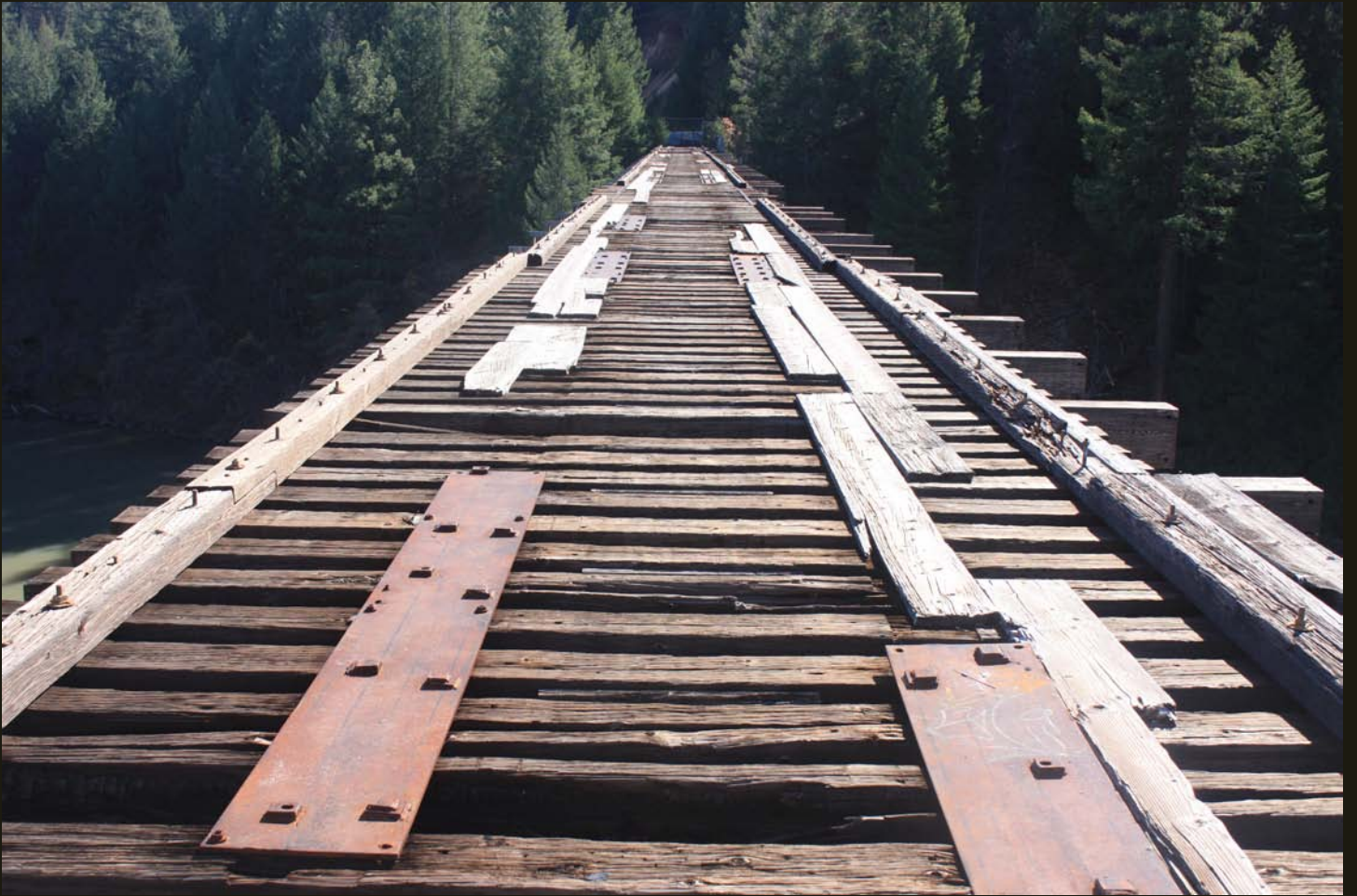
Top view of the trestle on the MR Burney Branch across Lake Britton; the trestle was built in 1954-55 and abandoned around 2005.
