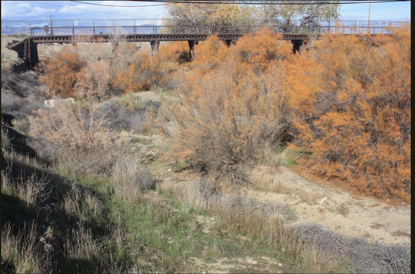
Another view of the SP Coalinga Branch (1888) where it crosses Gatos Creek just east of Coalinga.
