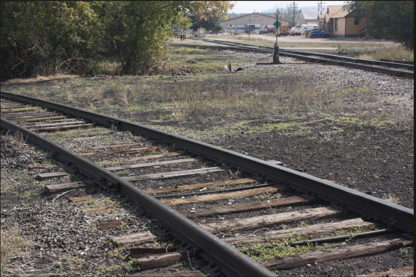
Southeastward view of the west branch of the wye (foreground), the track that emerges from the upper right edge of the photo is the D&RG San Juan Extension (1878n) mainline, the switch connects the mainline to the siding, and the depot is in the upper right.
