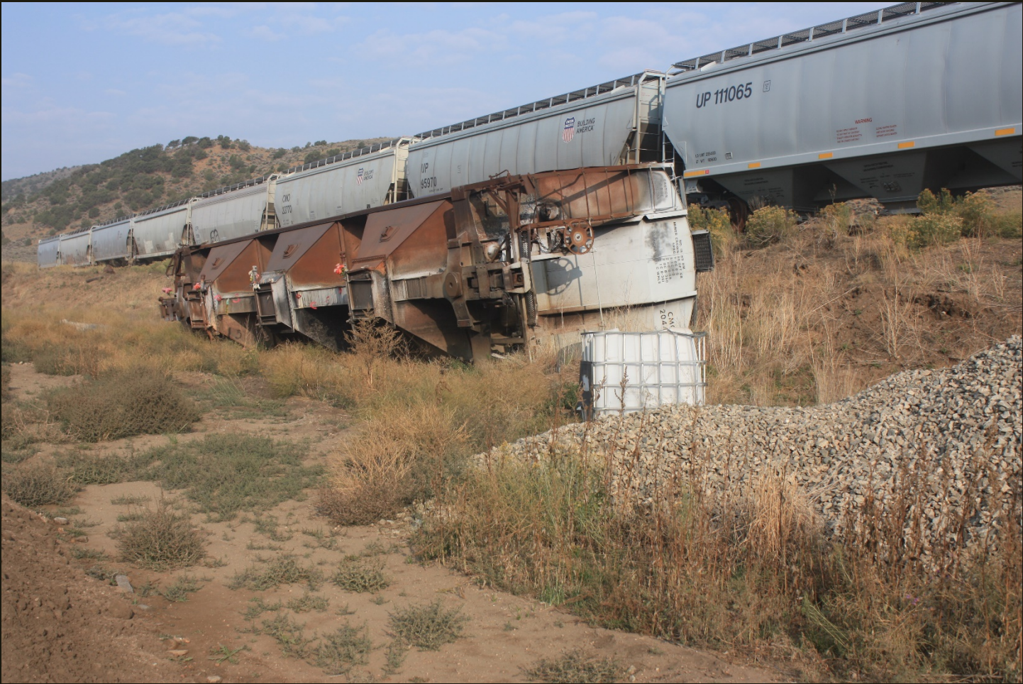
About 3,000 feet northeast the previous location, a hopper car has derailed and others are stored on a siding on the D&RG San Juan Extension (1899).
