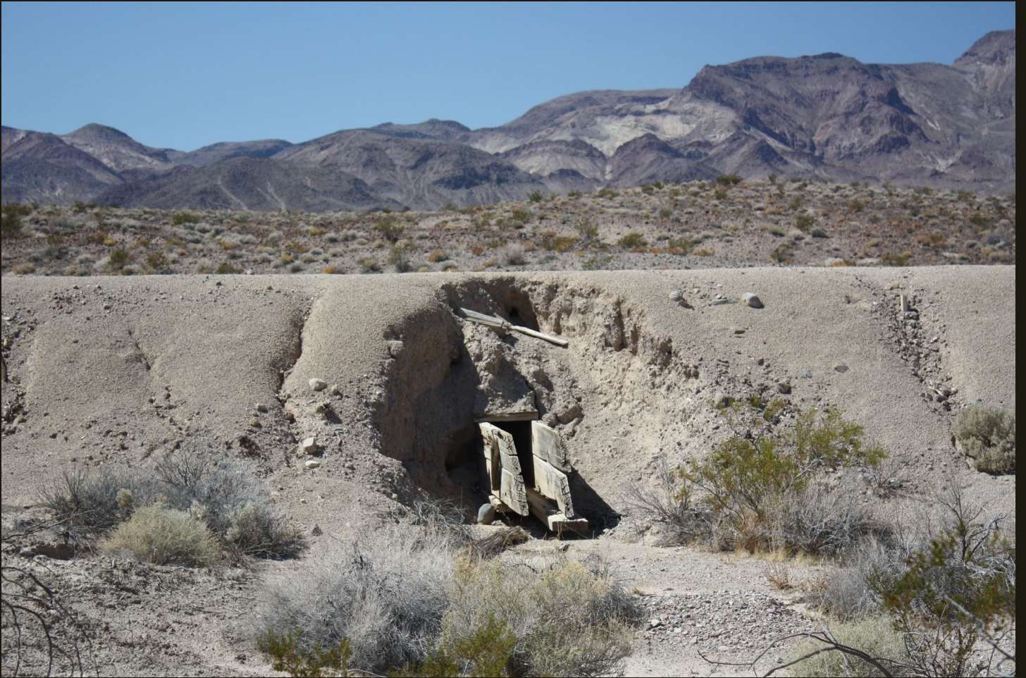
A wooden culvert on the T&T fill grade one mile north of the previous location.
