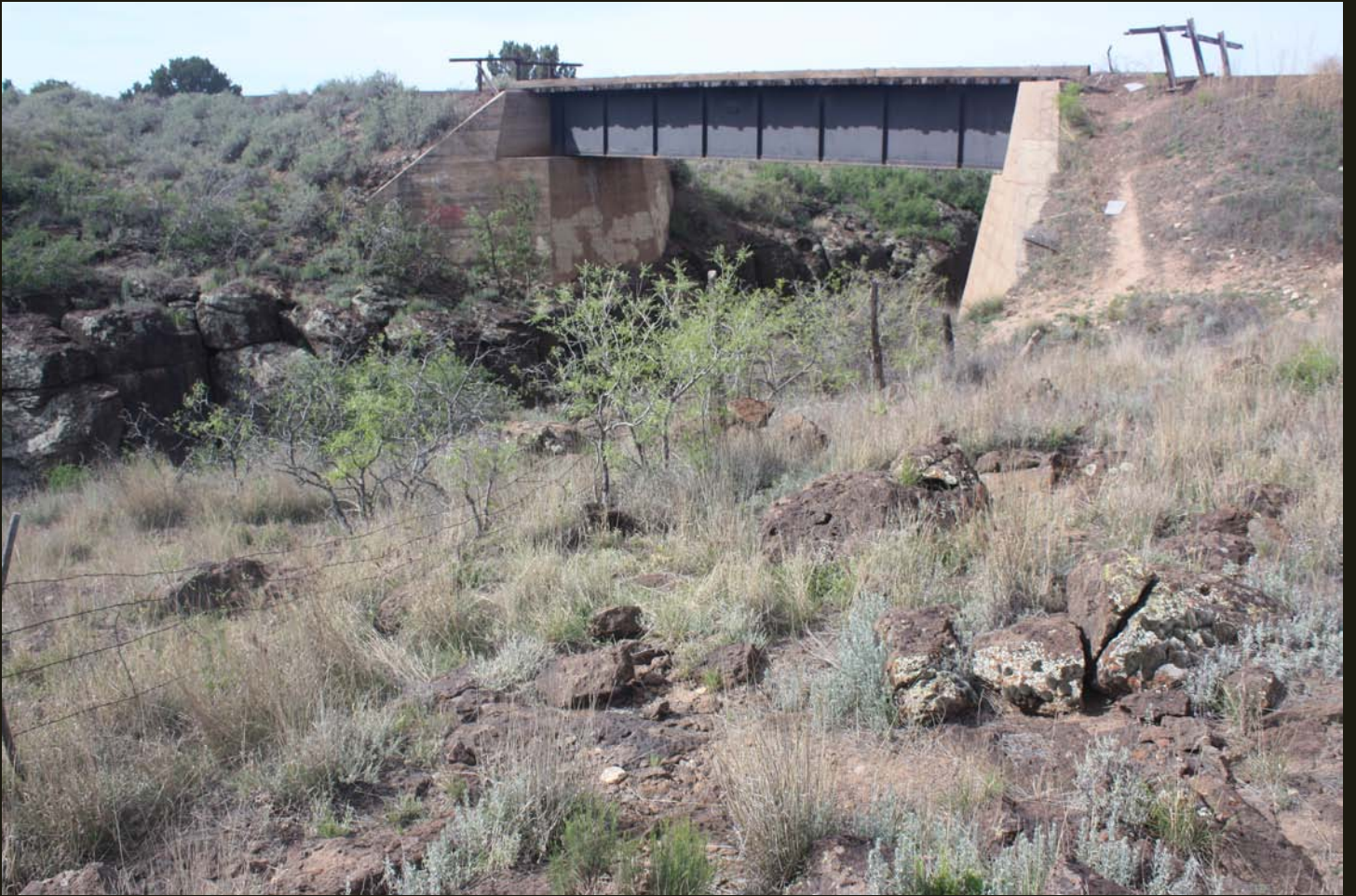
The SFP&P crosses the Verde River on this bridge 2 miles south of Paulden (previous photo).
