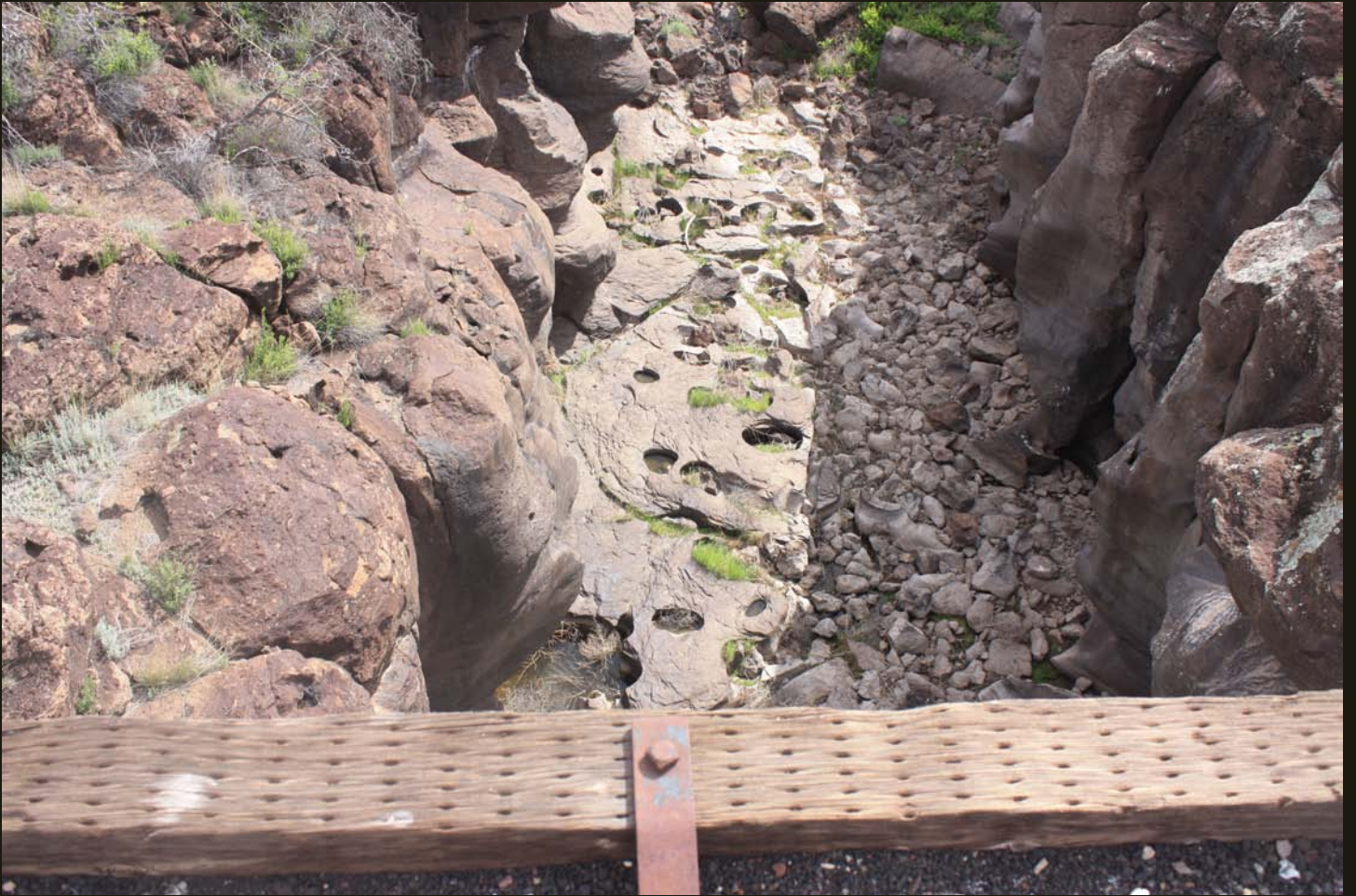
Same view as previous looking over the side of the bridge. Note the potholes eroded into the hard basalt by the Verde River during stronger flows.
