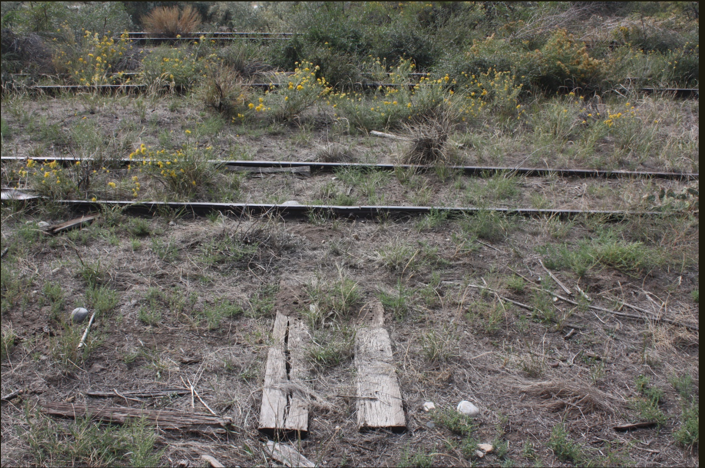
Southward view a few steps north of the previous location, showing two long ties for a former switch on the detached siding.
