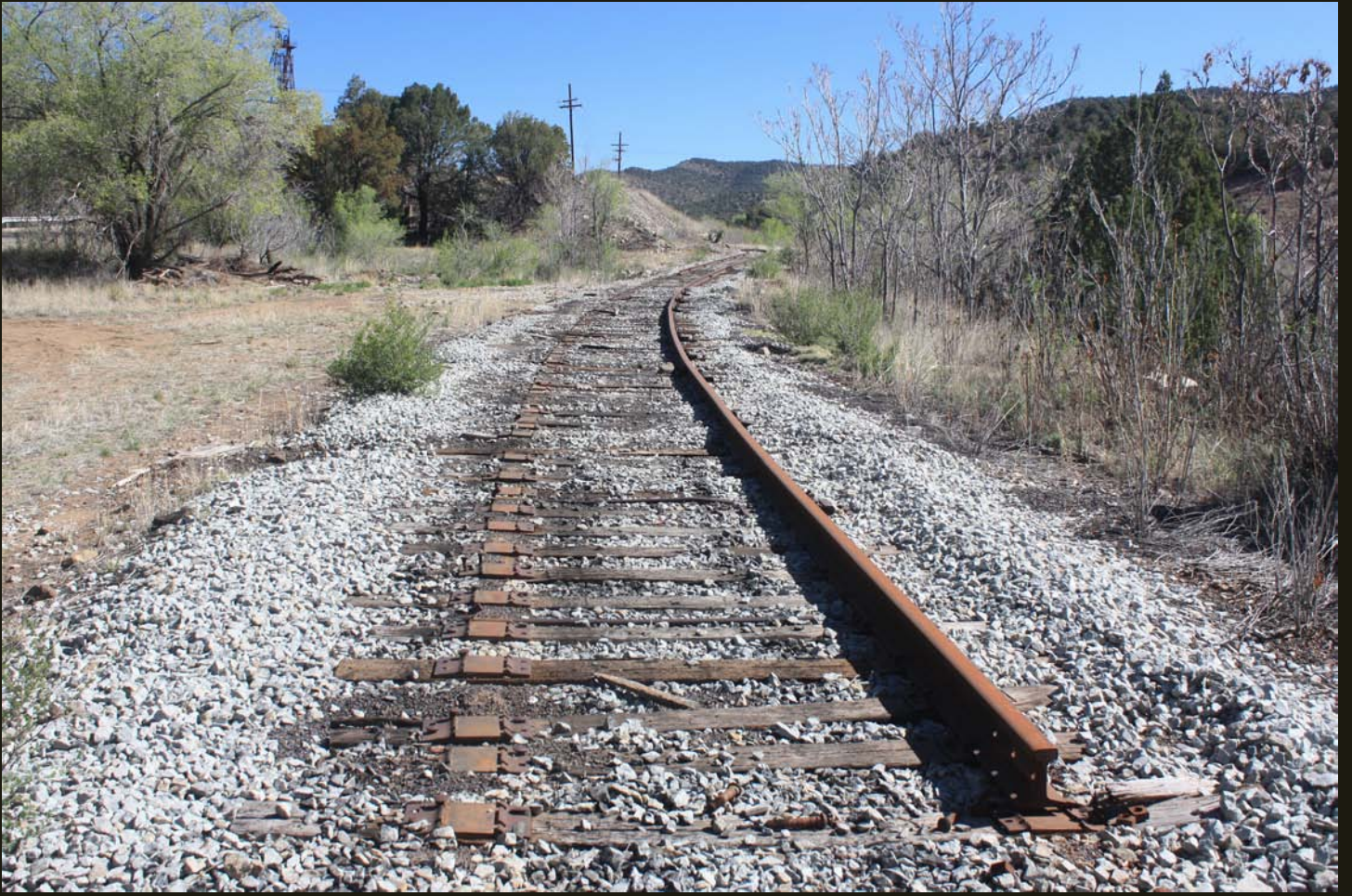
Missing rails just south of Hanover.
