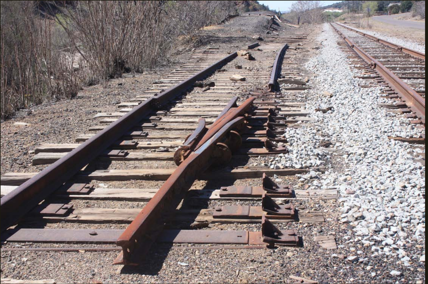
Part of a switch for a siding at the abandoned loading facility on the SC&N at Hanover.
