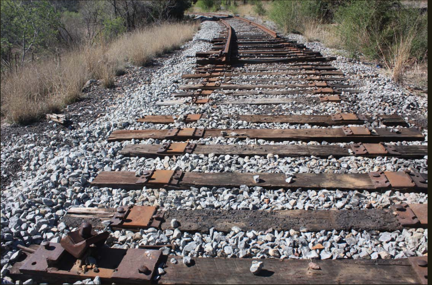
Another view of missing rails just south of Hanover.
