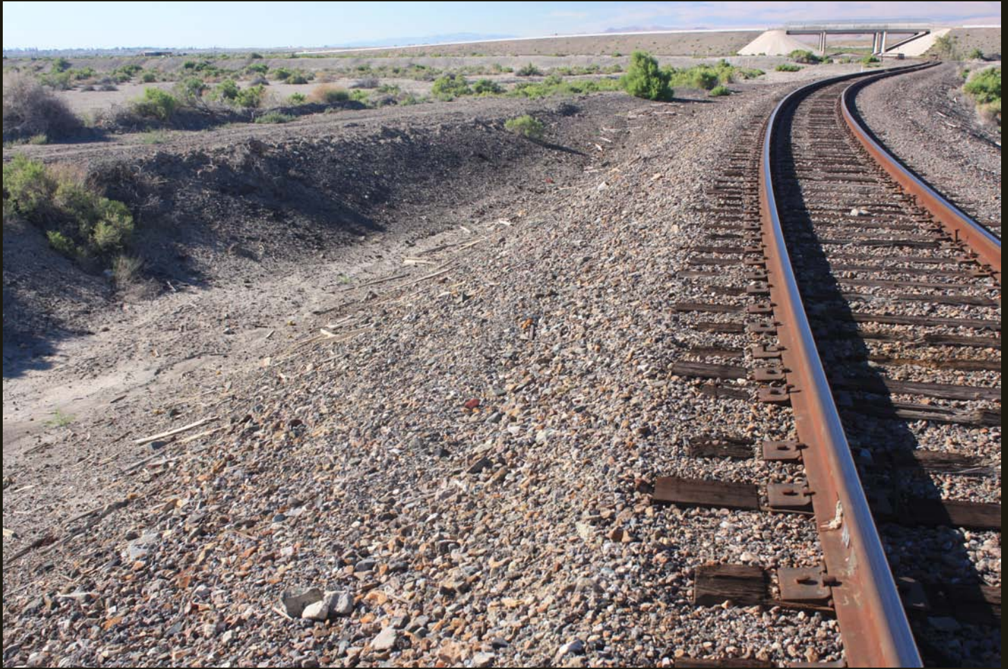
Southeastward view of the N&C Hazen Cutoff (1905), 900 feet southeast of the previous location. The fill grade for the abandoned eastern branch of the original wye is well preserved to the left. Note a small bridge with a small tree in the right distance and the U.S. Highway Alt 50 overpass behind it.
