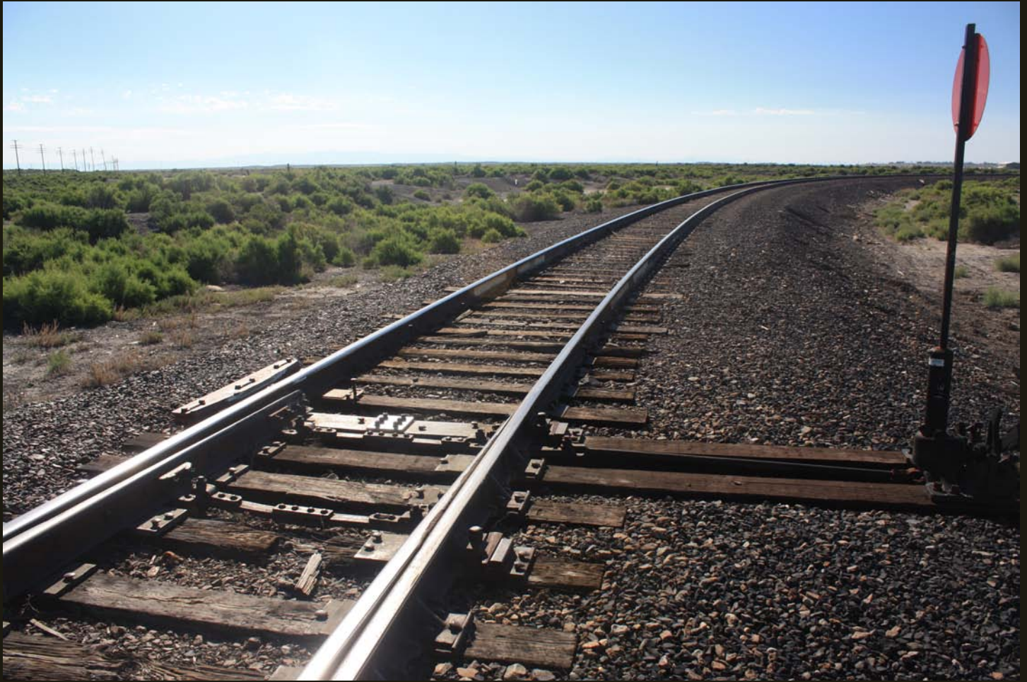
Southeastward view of the N&C Hazen Cutoff (1905) showing the same switch as the previous photo. Note the flat topography of the Carson Sink, the marshes and playas at the terminus of the Carson River and a remnant of Pleistocene Lake Lahontan. The fill grade for the abandoned eastern branch of the original wye is visible in the brush to the left.
