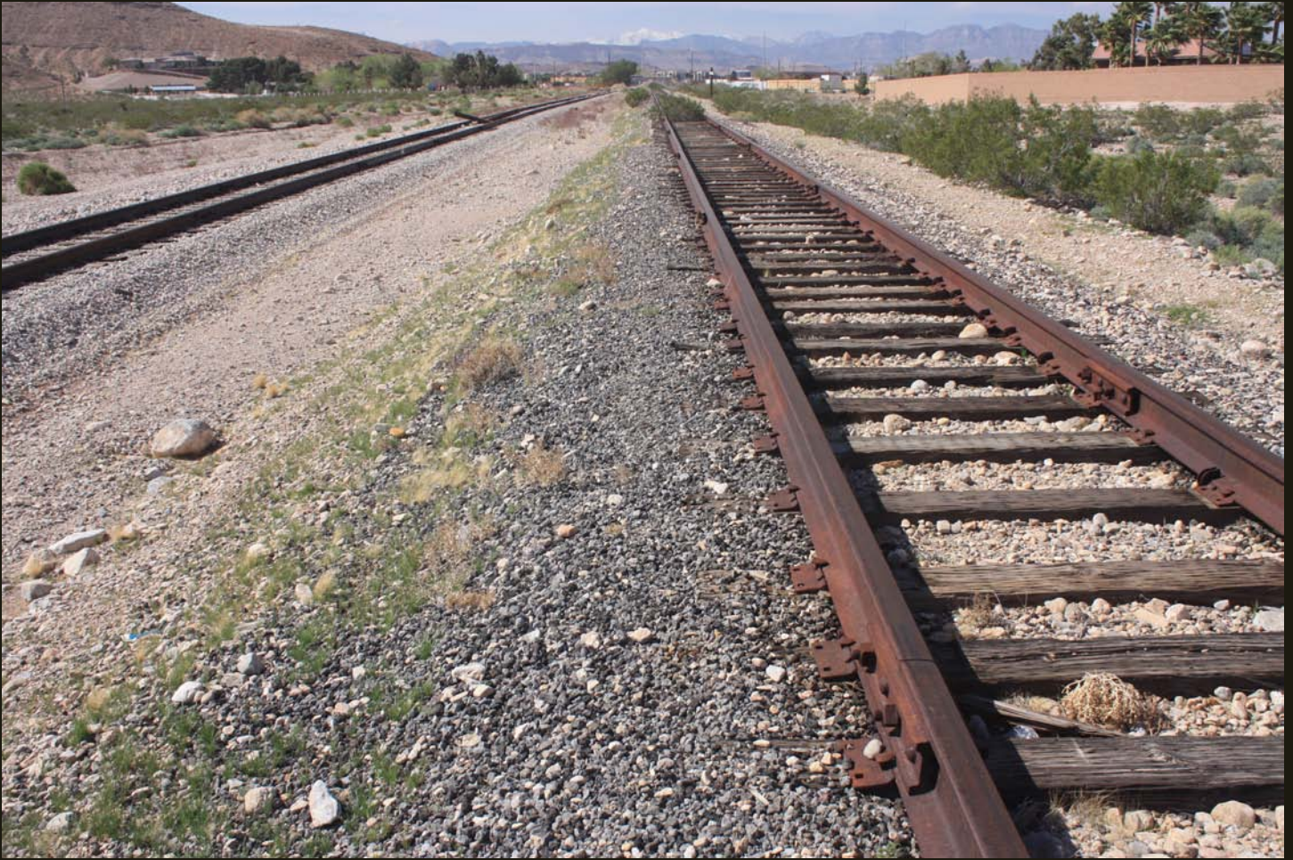
Westward view of the LA&SL Blue Diamond Branch and siding, west of the previous location and the stored cars. The track ends a quarter mile farther up the line.
