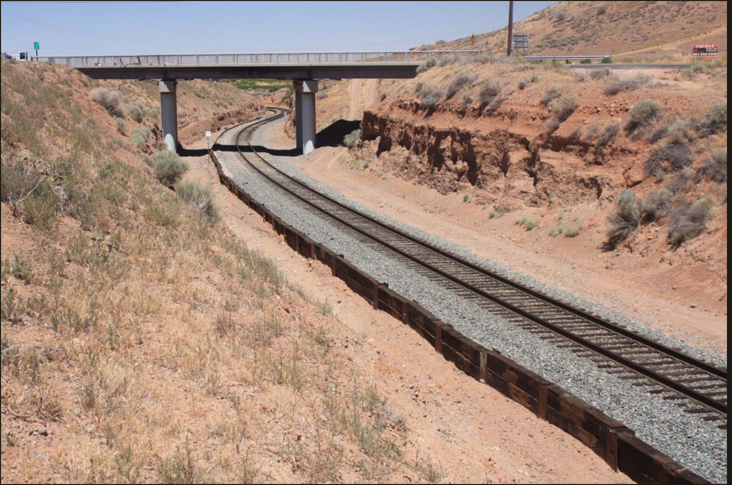
Same overpass as in the previous photo, showing a summit cut grade at Soledad Pass. The cut is in soft alluvium.
