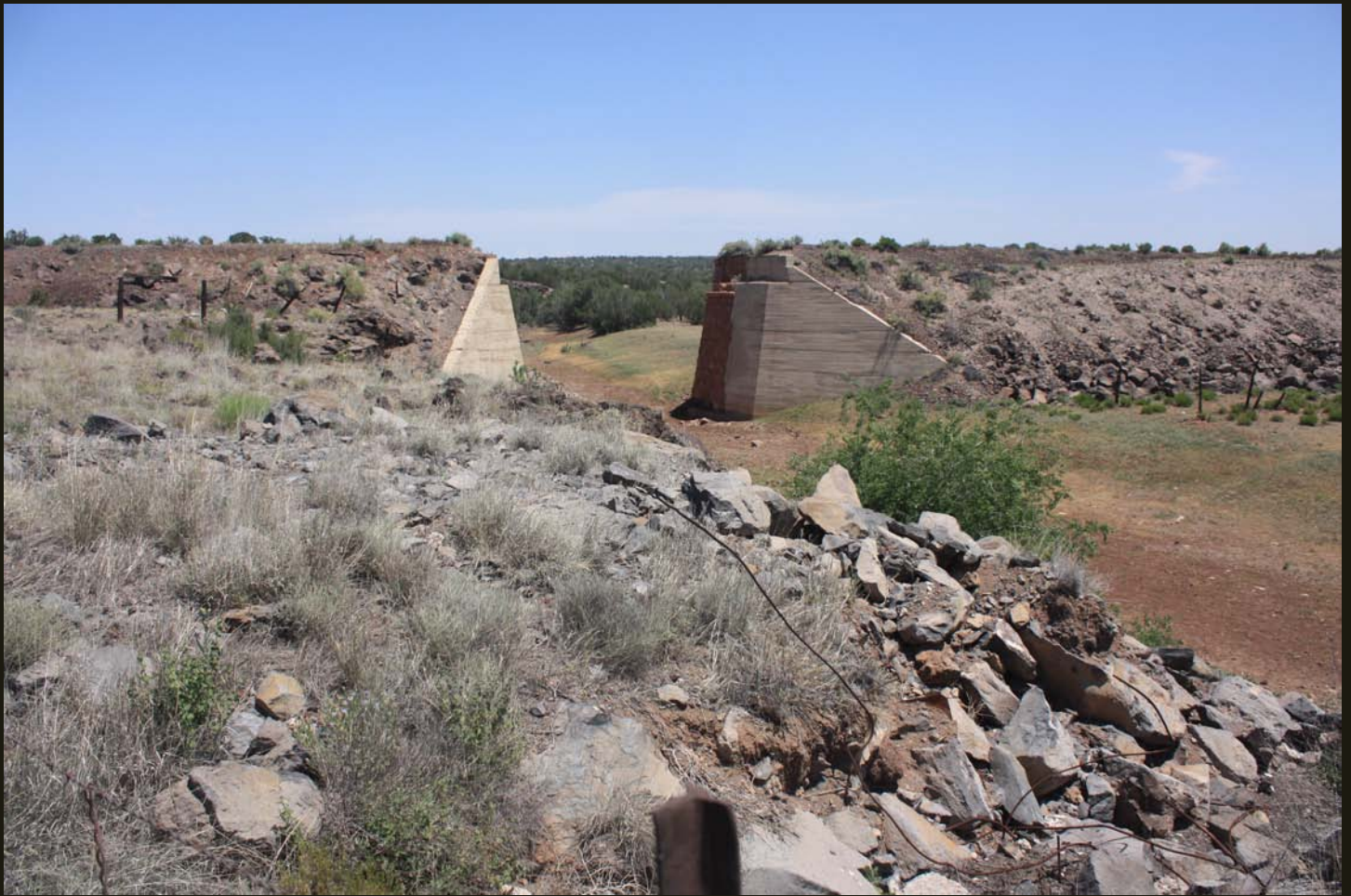
Abandoned bridge abutments on the abandoned A&P grade 5 miles west of Ash Fork. Note the red Coconino Sandstone, possibly original 1882 construction, and later concrete work, which pre-dates the 1960 abandonment of the line.
