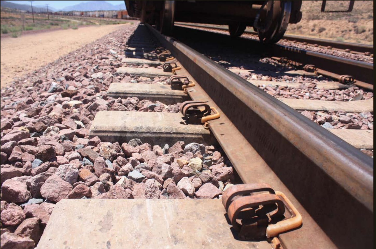
Same location as previous, showing detail of fasteners on concrete ties. No spikes here, golden or otherwise.
