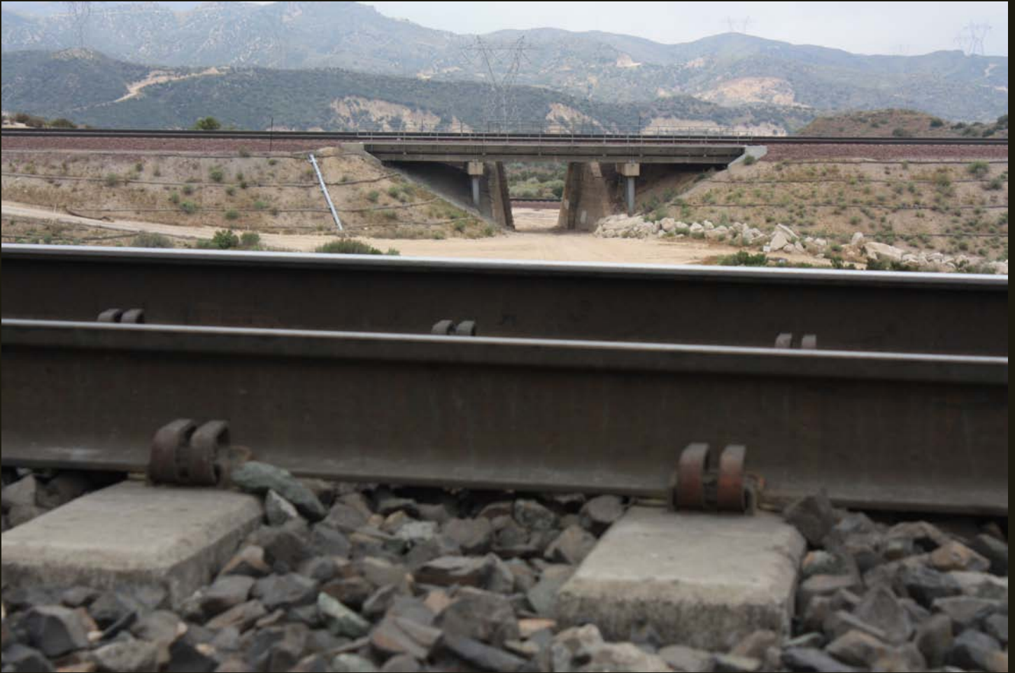
Southward view 3 miles southwest of Cajon Pass. The closest track is the SP (now UP) Palmdale Cutoff. The center grade is the 1913 AT&SF (now BNSF) double track. The farthest track, visible through the underpass, is the original CS (now BNSF) grade. Altogether four modern, concrete-tied tracks!
