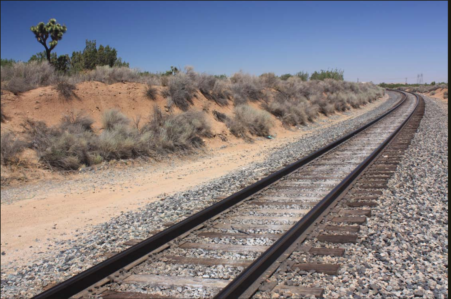
Northward view of the 1967 SP Palmdale Cutoff, where it curves left (northwest) toward Palmdale. Note the Joshua Tree at the southwestern limit of its desert range.
