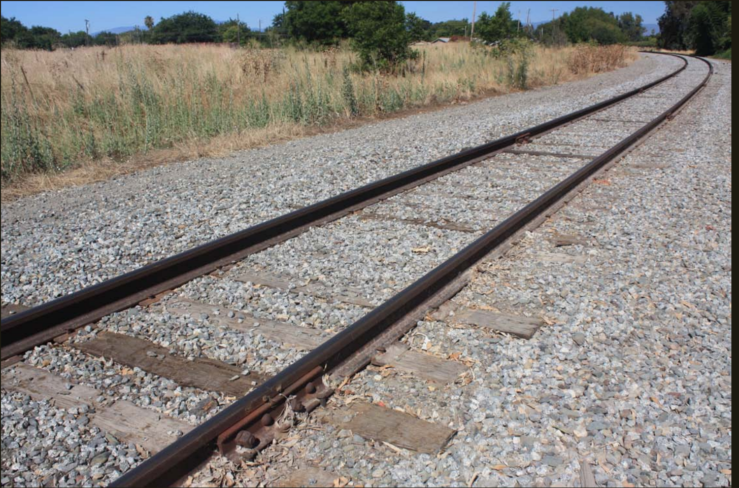
Northwestward view at same location as previous, the WS&M curving toward its due west course in the distance.
