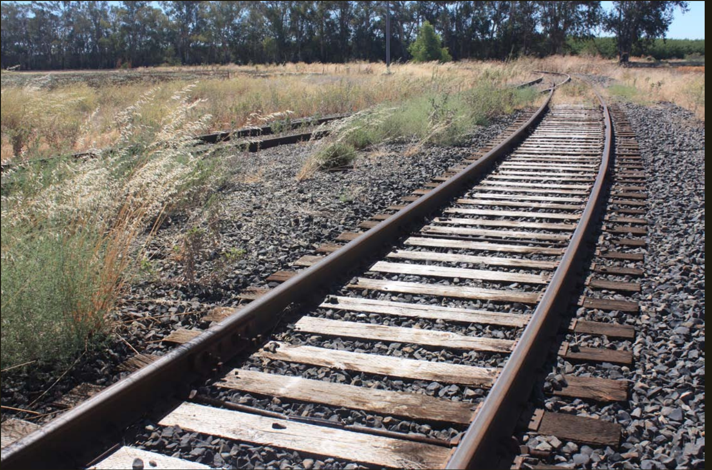
Southward view of the re-alignment where it curves to the north and splits off a siding.
