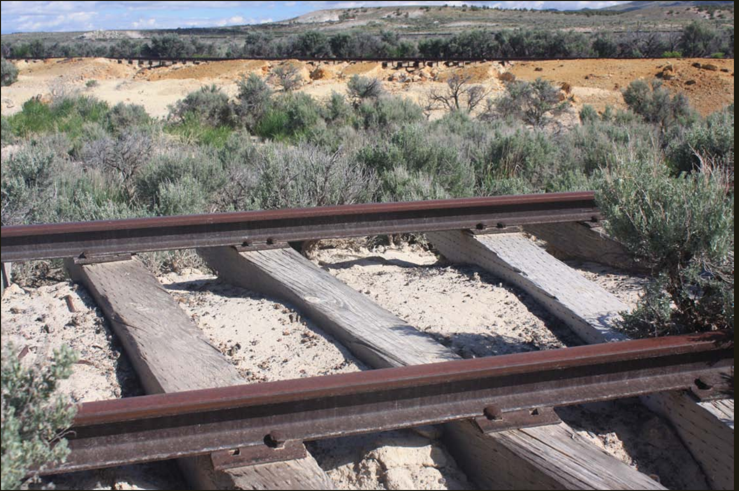
Now we are on the south branch of the Cobre turning wye looking northwestward at the south branch (foreground) and the north branch of the of the wye (middle distance).
