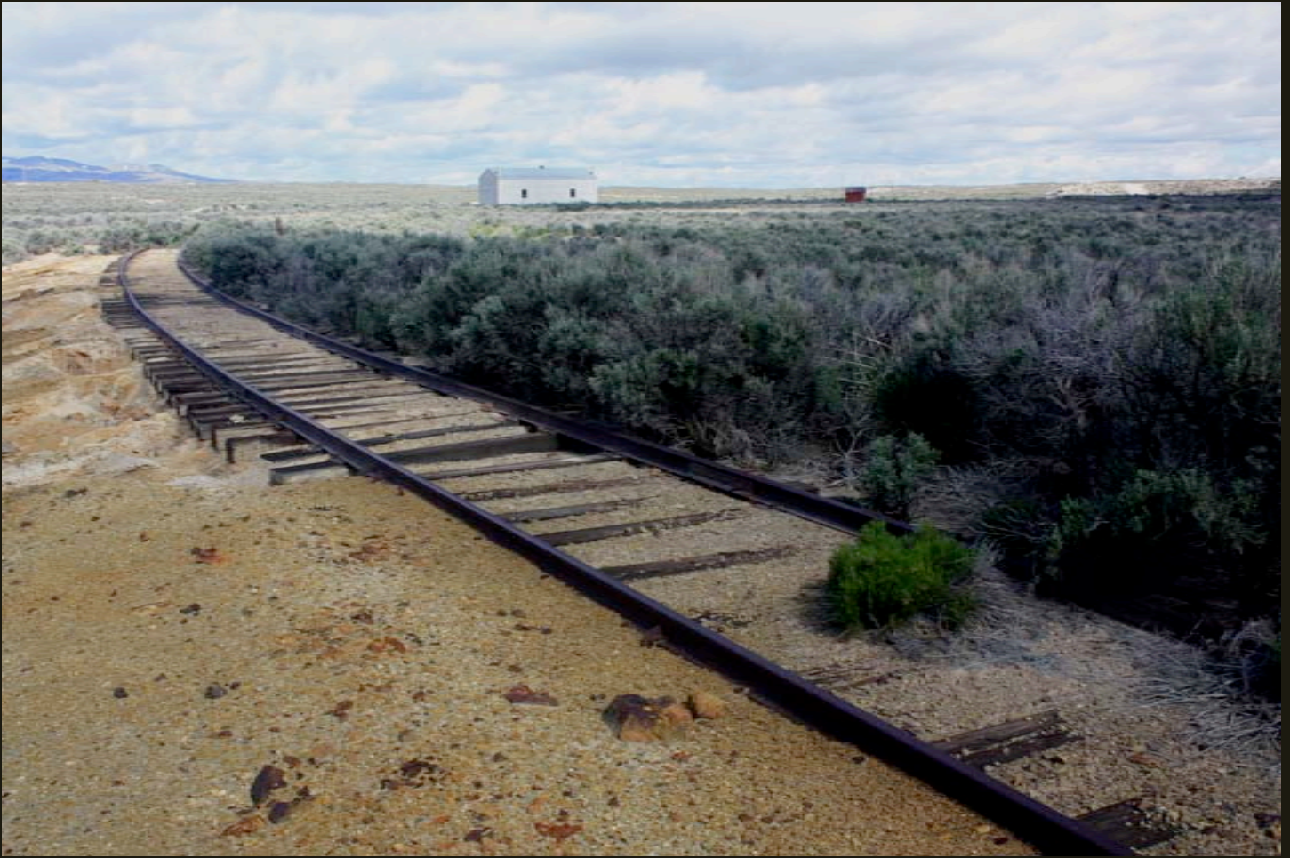
Westward view of the north branch of the turning wye. The yellow soil is iron oxide indicative of tailings used to repair the fill grade at this location and a few others around Cobre.
