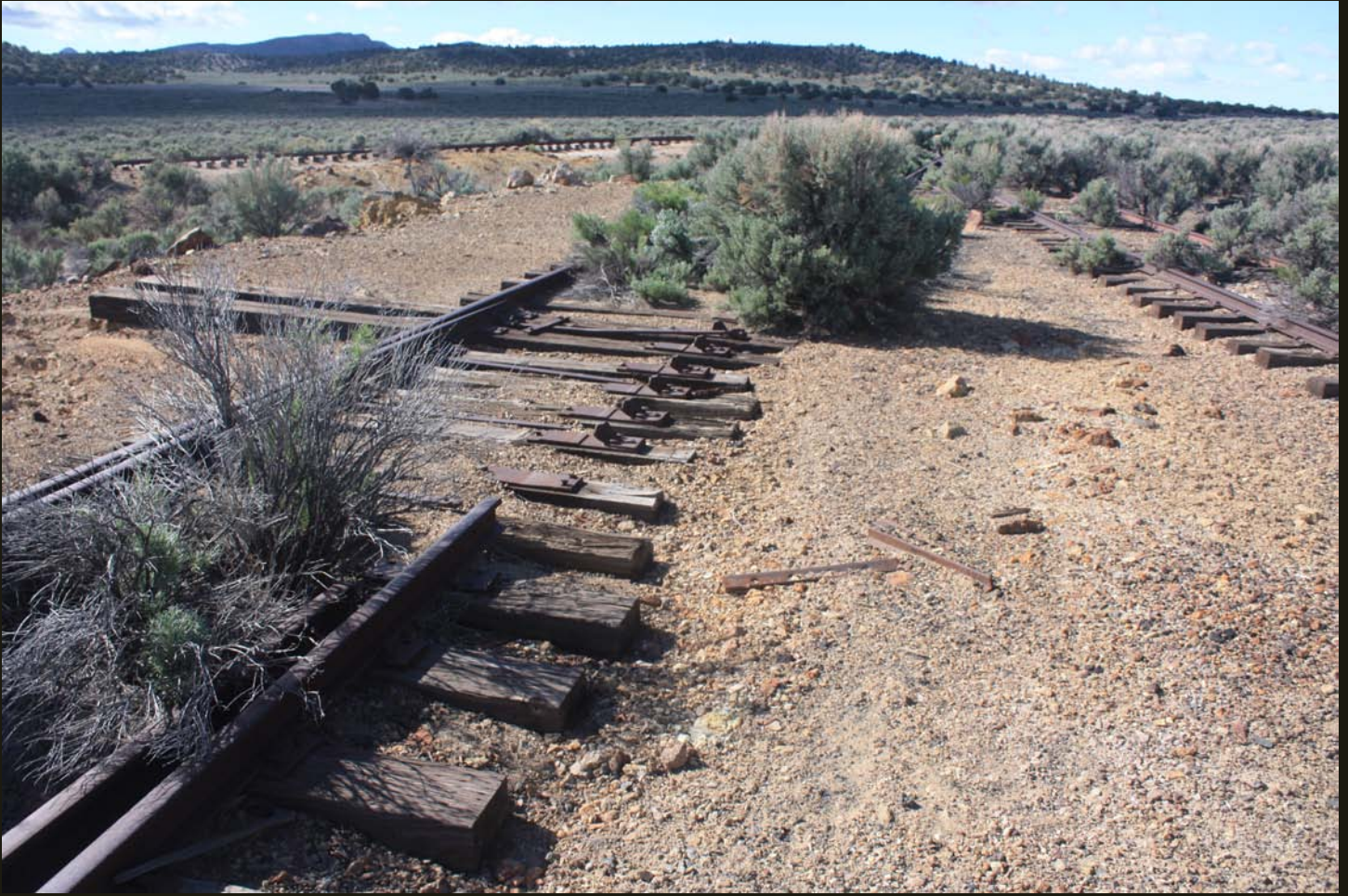
Southward view of the NN (1906), a few steps south of the previous location. The NN mainline is in the left foreground, with its switch to the siding for the north branch of the wye. The south branch of the wye is coming in from the left mid-distance. The track on the right leads back to the engine house and joins the NN mainline, now a single track, in the sagebrush ahead.
