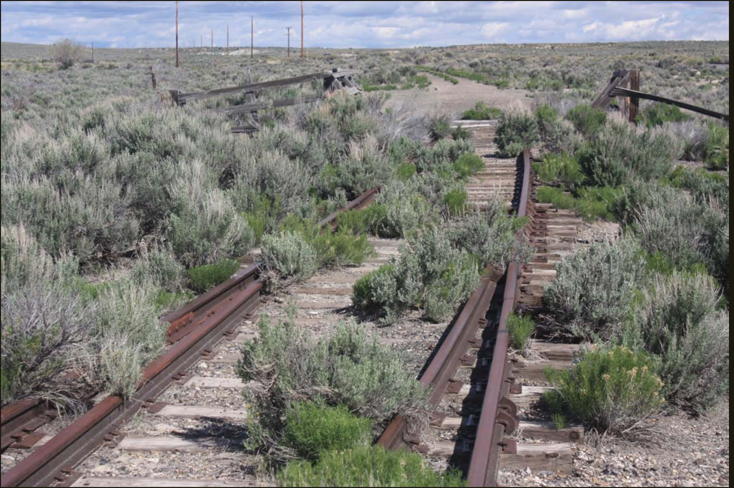
Northwestward view of the current end-of-track of the NN (1906) at Cobre. Same small bridge as previous photo. In the foreground, note the first split in the track as it enters the NN facilities at Cobre, which include two buildings, sidings, and a turning wye.
