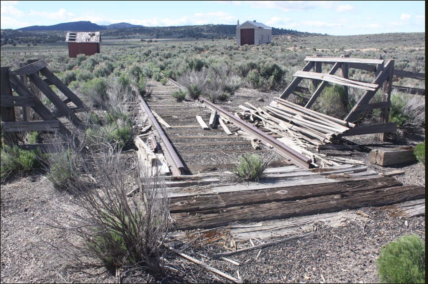
Southeastward view of the abandoned NN (1906) grade at Cobre. The track removal ends at this small bridge 1,600 feet southeast of the former connection to the NN siding; thus, 1,600 feet of track was removed.
