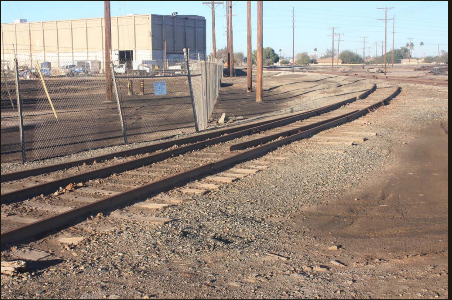
Westward view of the disconnected track to sidings south of the HI track.
