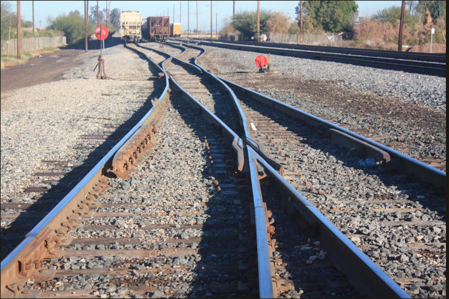
Northward view a few steps west of the previous location. The SP Inter-Cal line is the straight track to the right and the north branch of the SD&A (1919) wye is in the left foreground.
