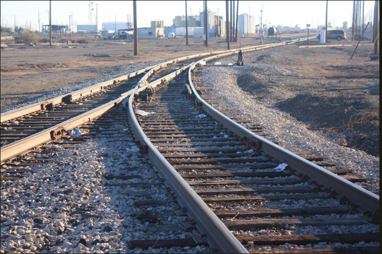
Eastward view of the HI (1904) wye. Note that just behind the switch for the wye, a track comes in from the right for sidings south of the track, but is disconnected from the mainline. Just beyond that, the track splits into active sidings for the facilities in the center distance. Current end of the track is about 2 miles east of this location.
