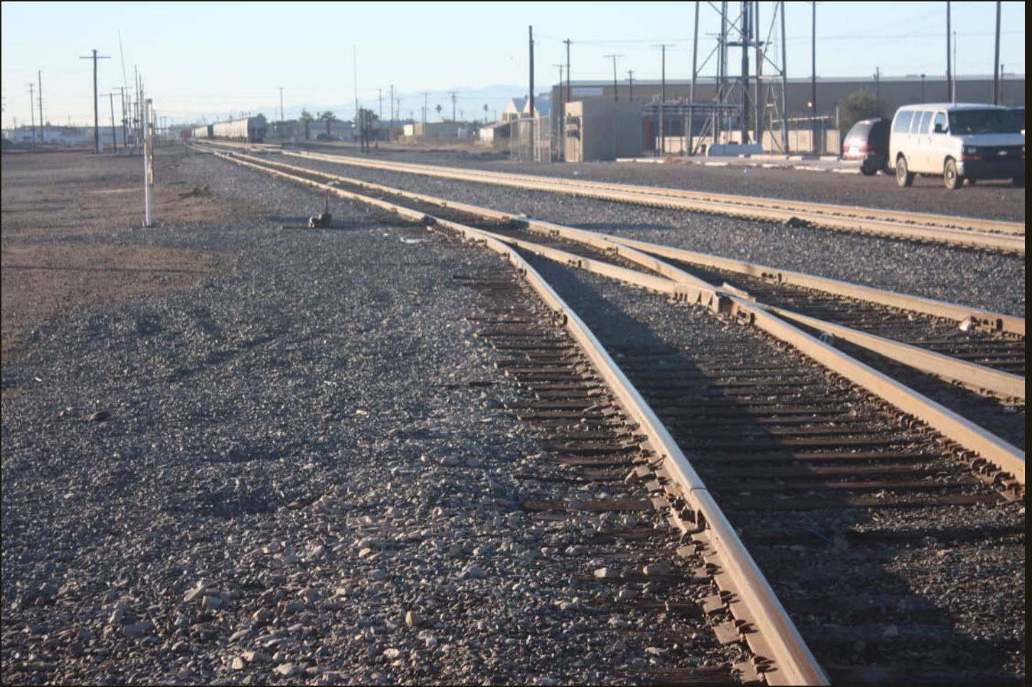
Southward view of the SP Inter-Cal (1904) at the same location as previous. The switch for the south branch of the HI (1904) wye is in foreground.
