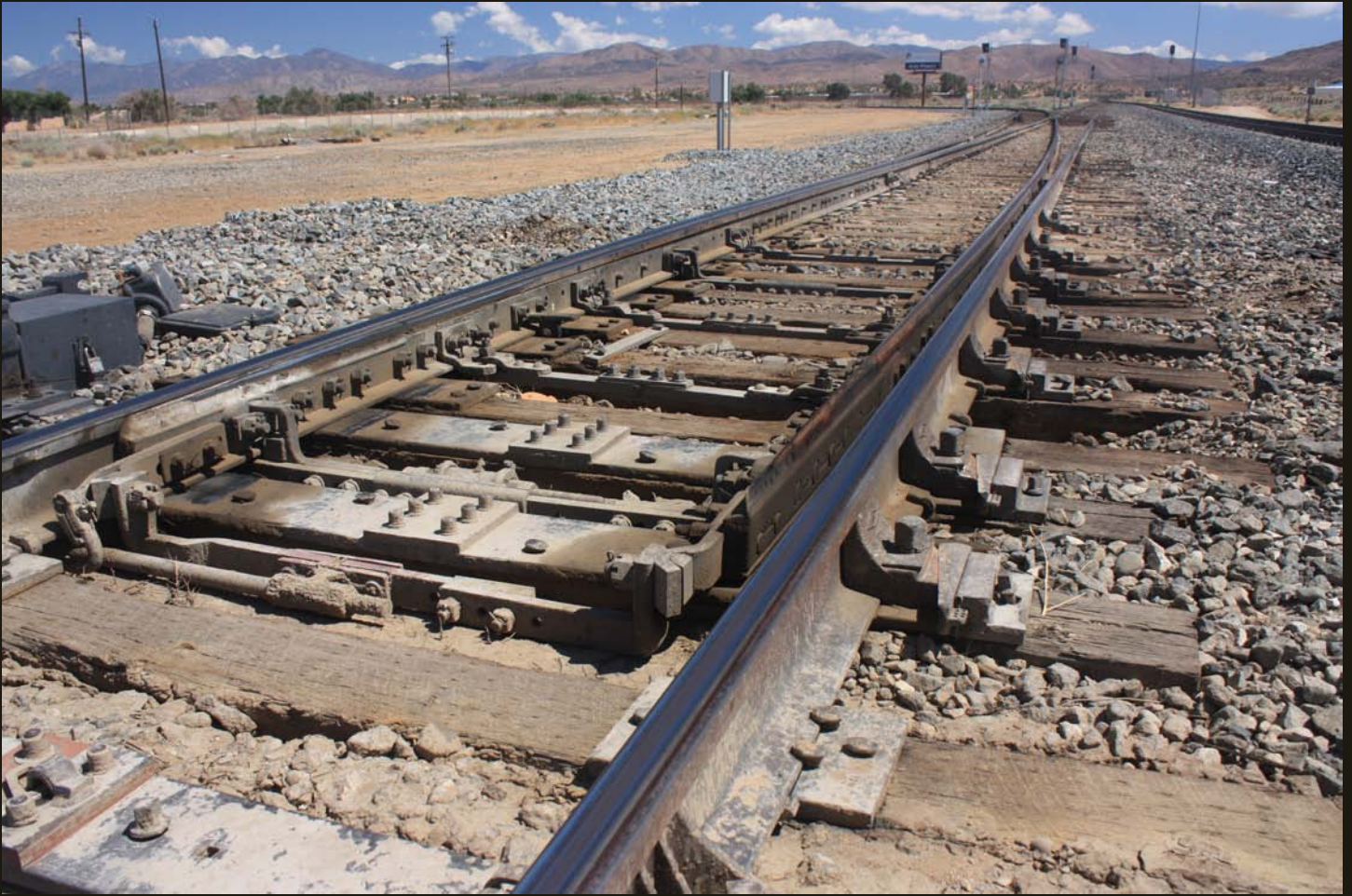
Southward view of the switch for the Palmdale Cutoff, with the SP (now UP) mainline on the far right. There is no wye, only this one switch, because this is a cutoff and there is no reason for a complete wye.
