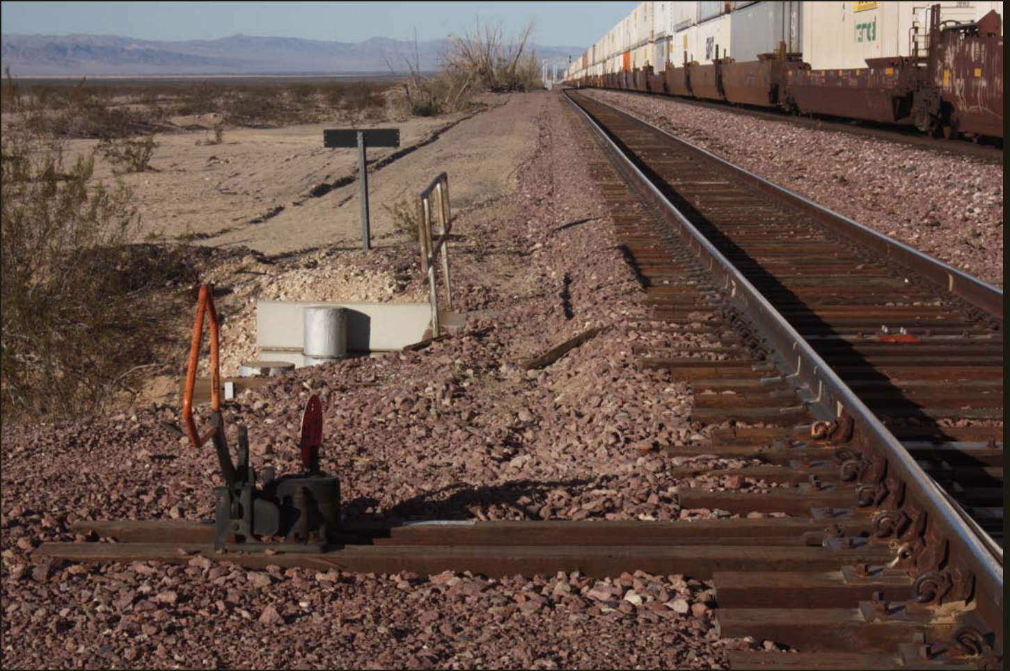
Westward view just west of the previous photo, with the same “new” siding seen in the previous photo. The switch in the foreground is the first switch for the Cadiz yard.
