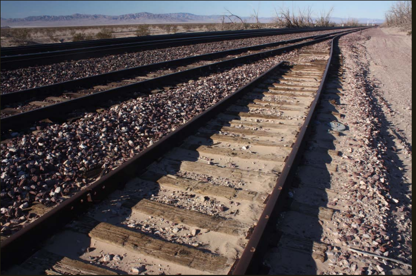
Westward view at the same location as the previous photo, with the old siding and switch to a second old siding in the foreground; the latter is physically disconnected from the line, as seen here, and extends only about 300 feet to the east.
