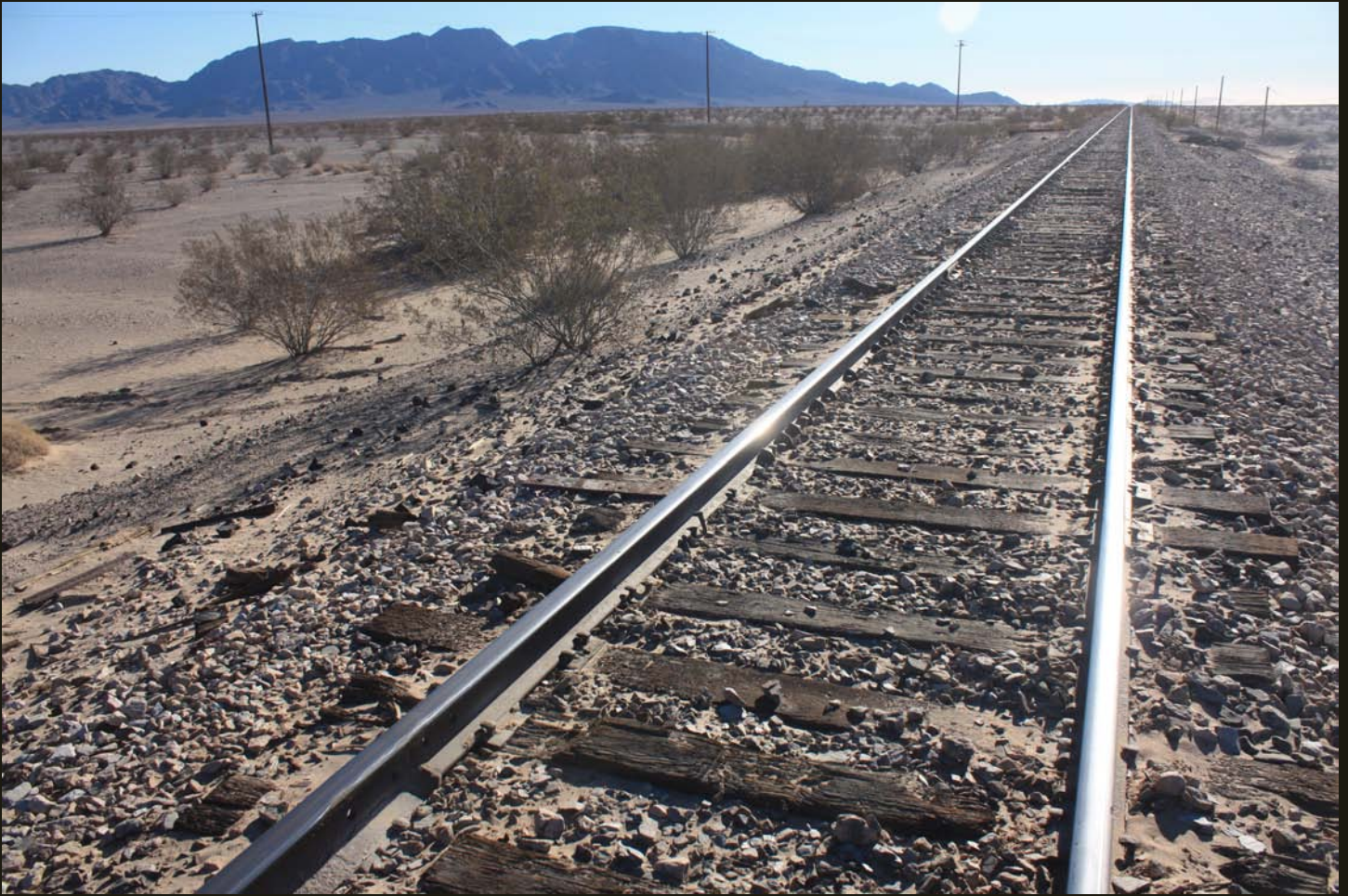
Southeastward view of the A&C (1910), same location as previous, as it heads across the desert to Arizona.
