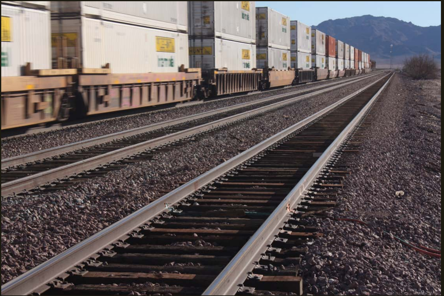
Eastward view at same location as previous. Note that the siding (far right track) merges onto the BNSF main line in the distance. East of that point the double track heads east to New Mexico and beyond.
