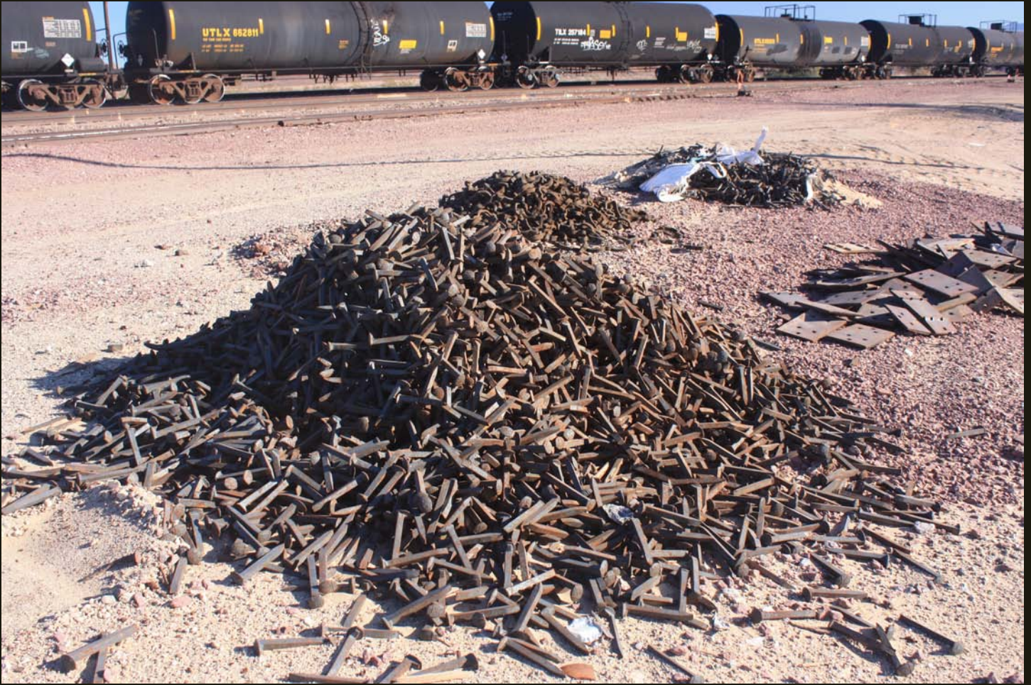
Scrap spikes and plates at the Cadiz yard. Note that the sidings are beginning to converge at the right (east) end of the Cadiz yard.
