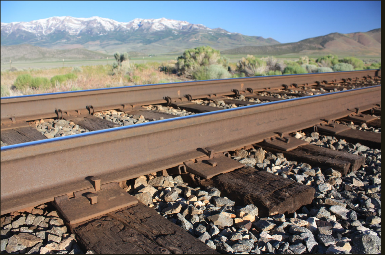
Westward view of the WP (1909) about 10 miles south of Wells, with the once-glaciated East Humboldt Range in the background.
