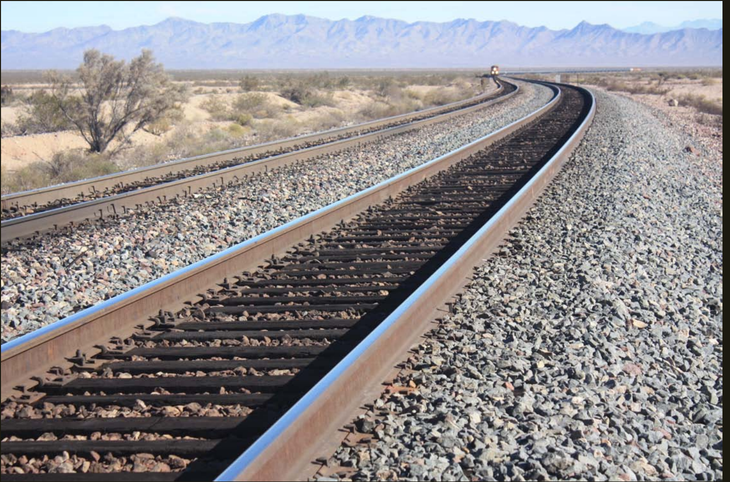
Eastward view of the same BNSF oil tanker train as the previous photo on the SP (1883) Needles Branch (now BNSF Southern Transcon).
