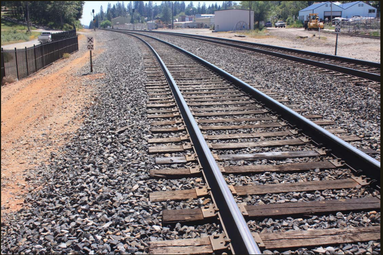
Southwestward view of the double-track CP (1869), 2,000 feet northeast of the Colfax depot. Note the short spur to the right with a parked track maintenance vehicle. According to topo maps from 1887 and 1932, the NCNG ran parallel to the CP (SP in 1887) on the road to the left (southeast), where the truck is driving; that road is appropriately called Narrow Gauge Road.
